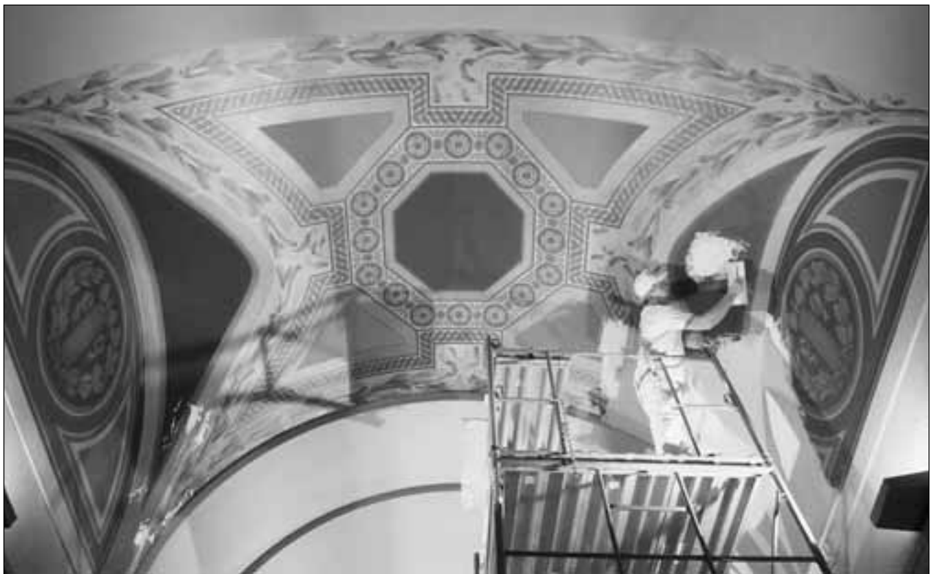
Rick Dahm of Luczak Brothers, Inc., applies a layer of gypsum plaster to the ceiling on the third floor of the Capitol Jan.11.
