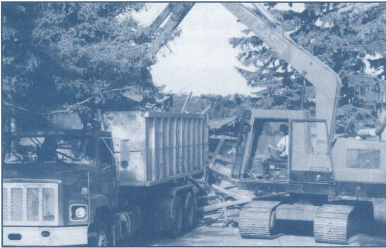
The Building Demolition crew loads building debris into one of their new roll-off trucks.
