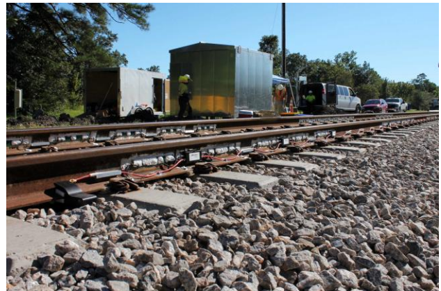
Figure 15: Example Truck Hunting Detector System with Strain Gauges
