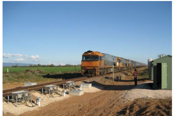
Figure 17: Truck Bogie Optical Geometry Inspection System
