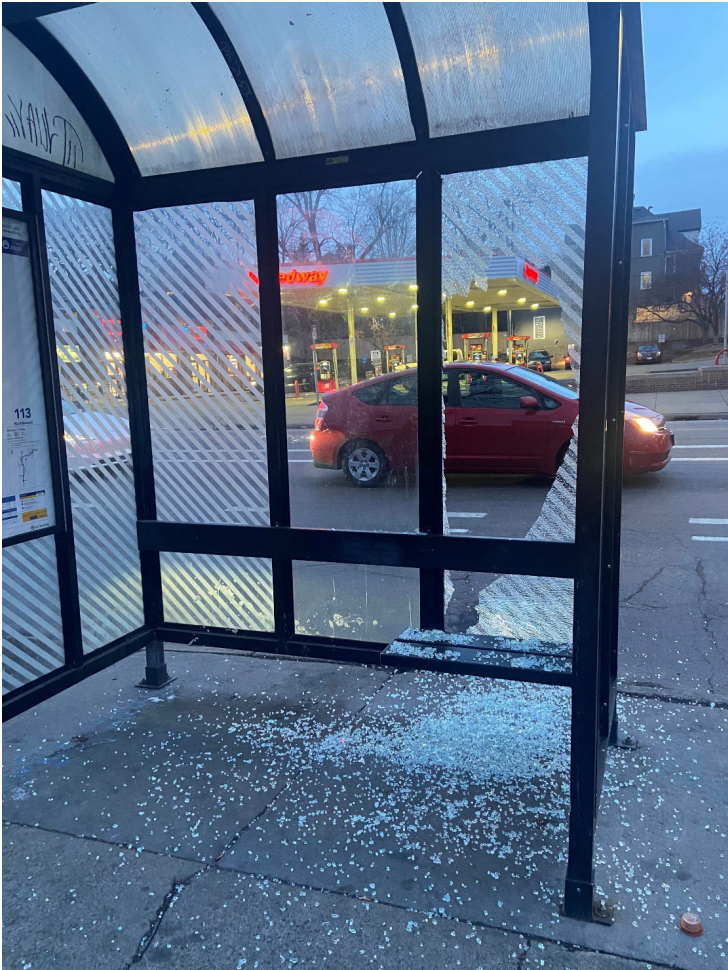
Figure 8: Broken Shelter Glass
