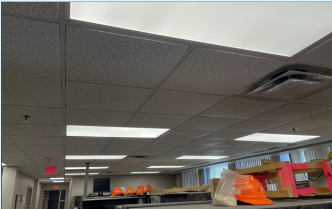
📷 Improved Lighting at Metro Oakdale Headquarters. Image courtesy of Mark Moehlenbrock, MnDOT.
