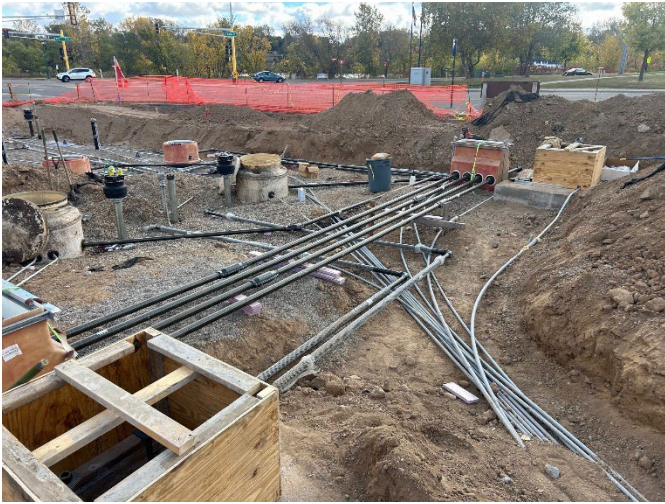
Photo 3. Photo taken during the construction of the new fueling equipment at The Corner Store, located in Inver Grove Heights.
