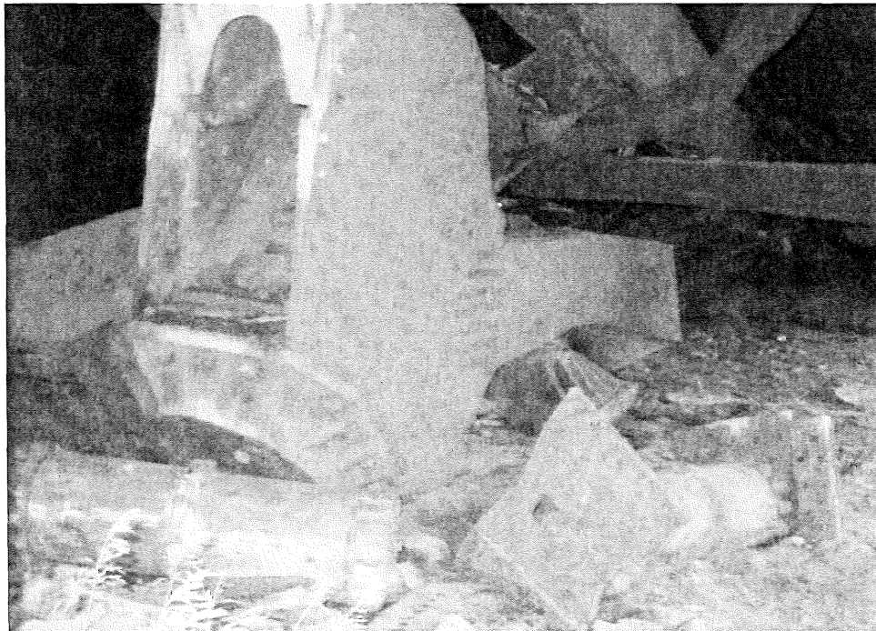
Figure 4.53. Post-collapse location of LIE, upper casting and north and center rollers.
