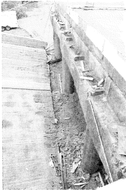
Figure 4.64. Collapse of the southbound lanes of Span 11 at Pier 11.
