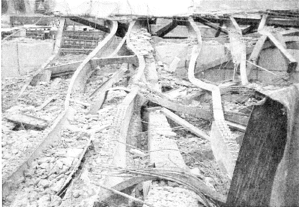
Figure 4.52. Typical distortion of stringers (Nodes 2' to 4', southbound lanes).
