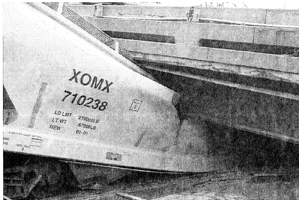
Figure 4.77. Railcar crushed under north approach.
