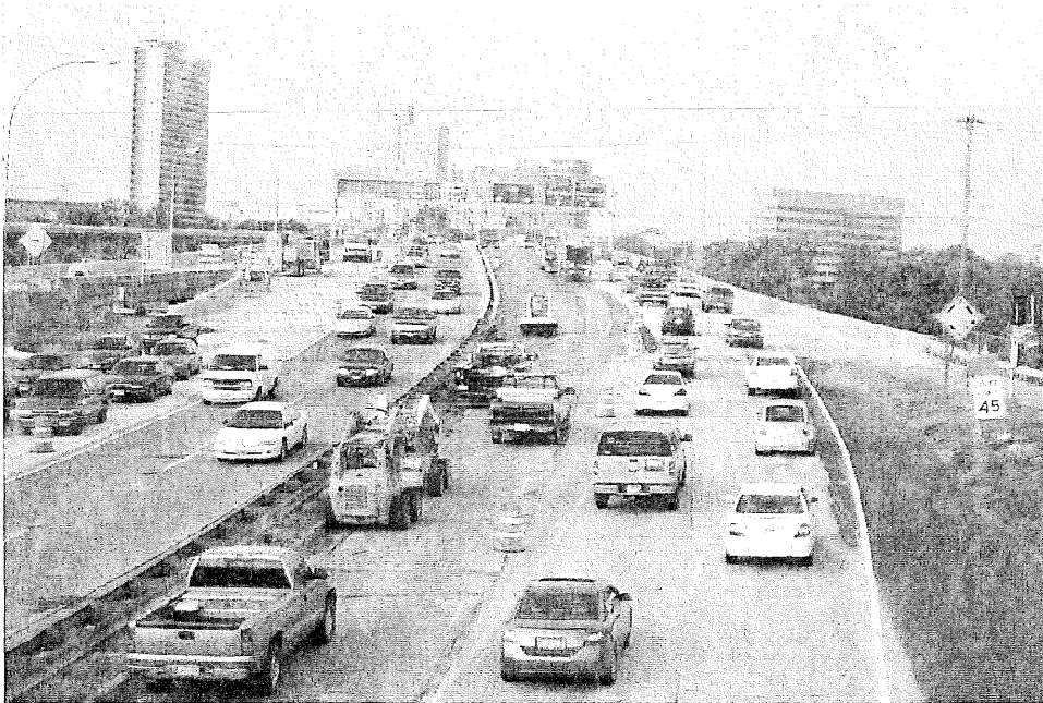
Figure 2.20. Ongoing overlay work by PCI during July 2007. Note milling operations in southbound inside lanes (view looking south).
