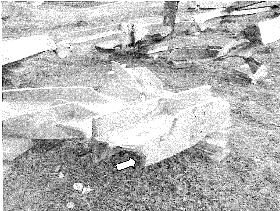
Figure 4.75. Fracture in the top chord of FT10 near Node U10 East. View looking west.
