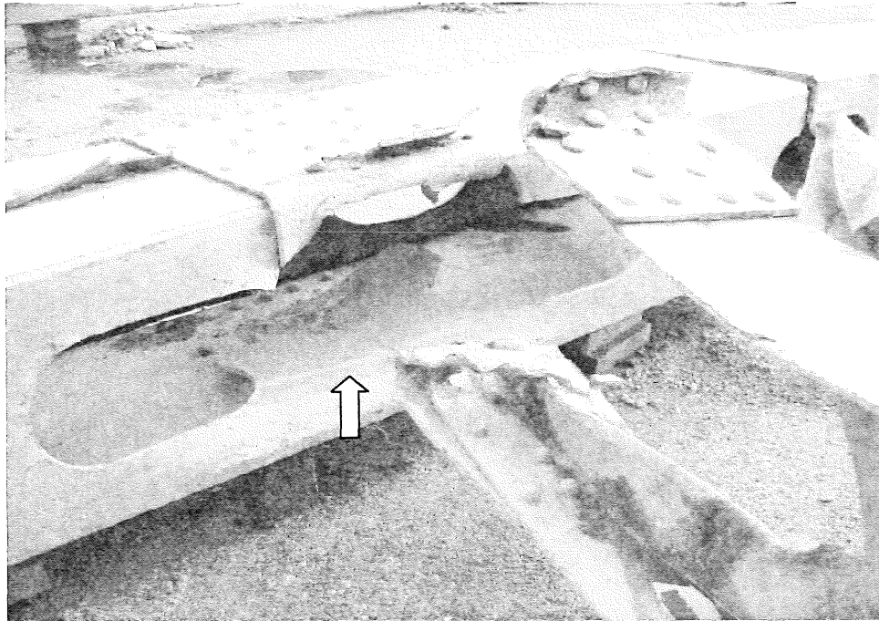
Figure 4.22. Impact damage on top cover plate of lower chord at L12'E.
