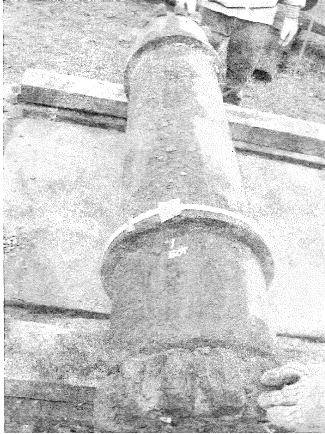
Figure 4.56. Corrosion on bottom of roller of west bearing at Pier 6.
