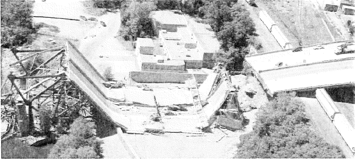
Figure 4.17. Post-collapse view of Span 8 looking west.
