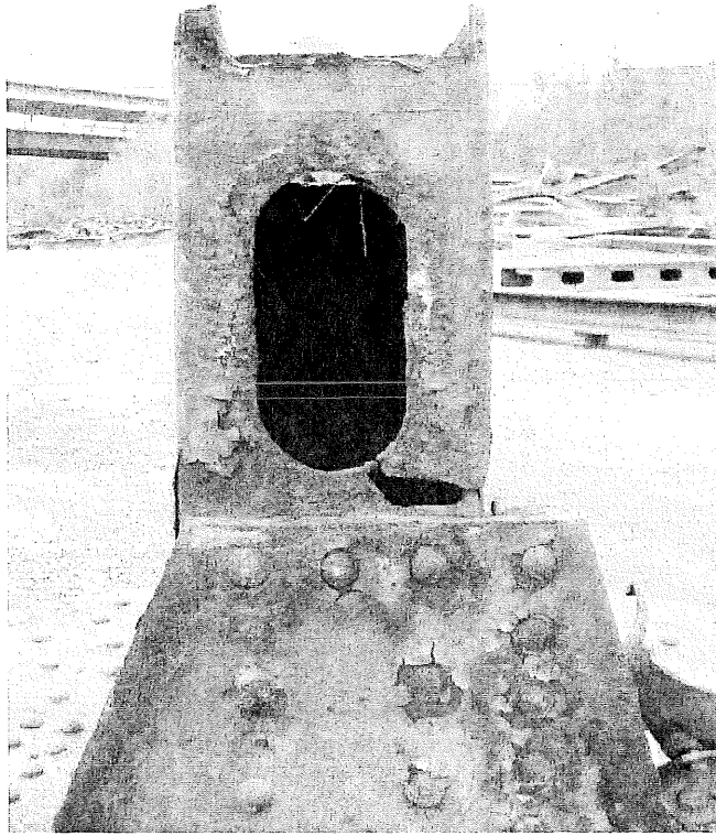
Figure 4.50. Corrosion on bottom of lower sway horizontal CL8'-L8'E at L8'E.
