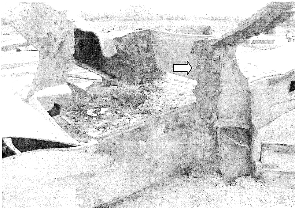
Figure 4.51. Corrosion on top connection plate to upper lateral at U4'E.
