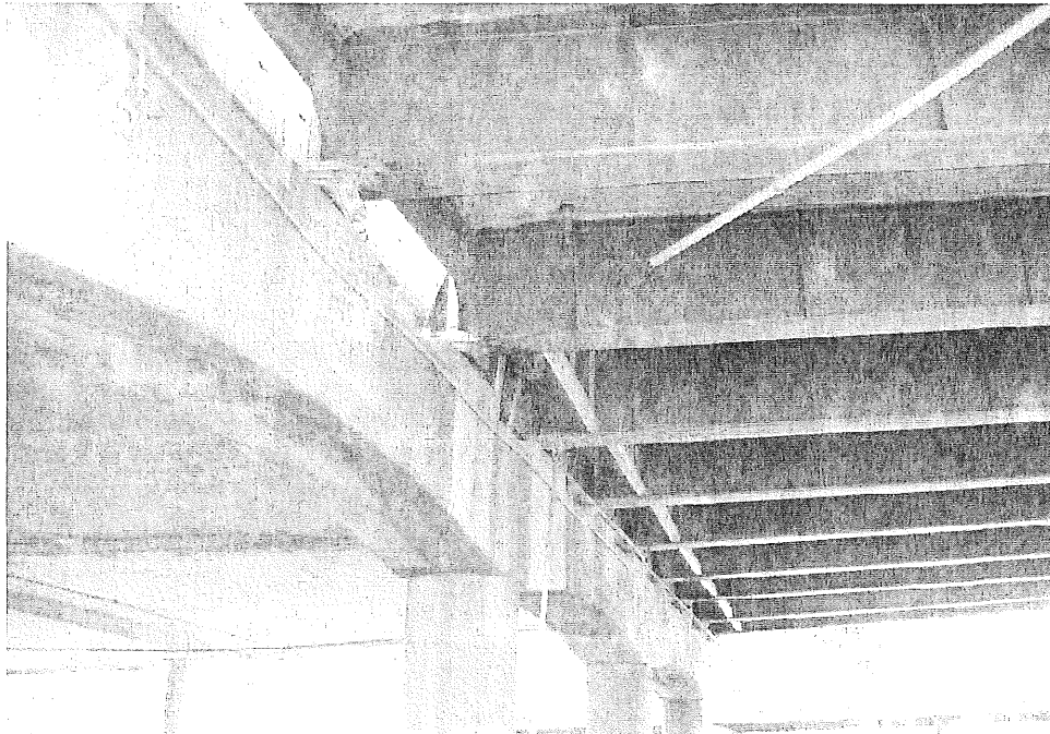
Figure 4.66. Southward displacement of bearings of the northbound lanes at Pier 11.
