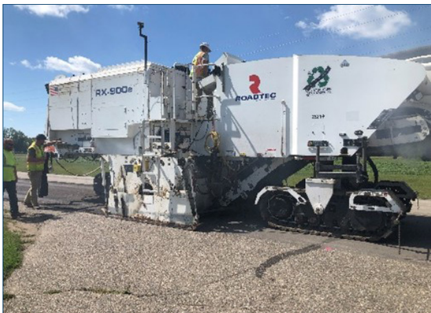
📷 Micromilling equipment used in resurfacing TH 28 near Swanville. Photo courtesy of Joel Ullring, MnDOT.
