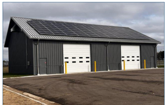
☒ Recently installed solar panels atop the Northfield Truck Station. Photo courtesy of Brian Ivers, MnDOT
