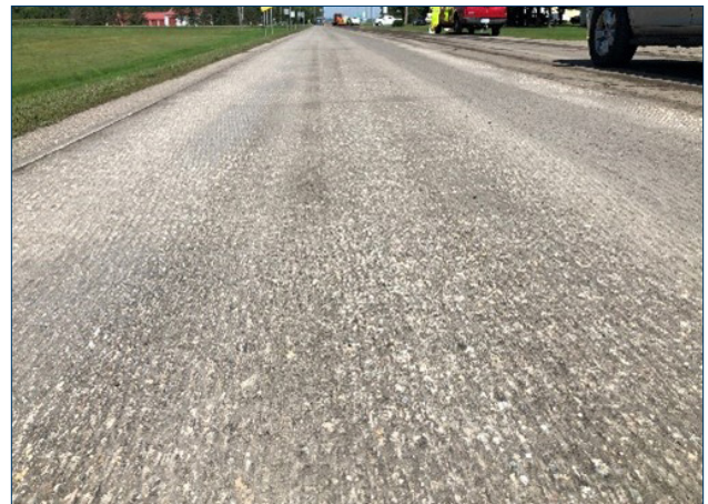
📷 Micromilled roadway surface of TH 28 near Swanville. Photo courtesy of Joel Ullring, MnDOT.
