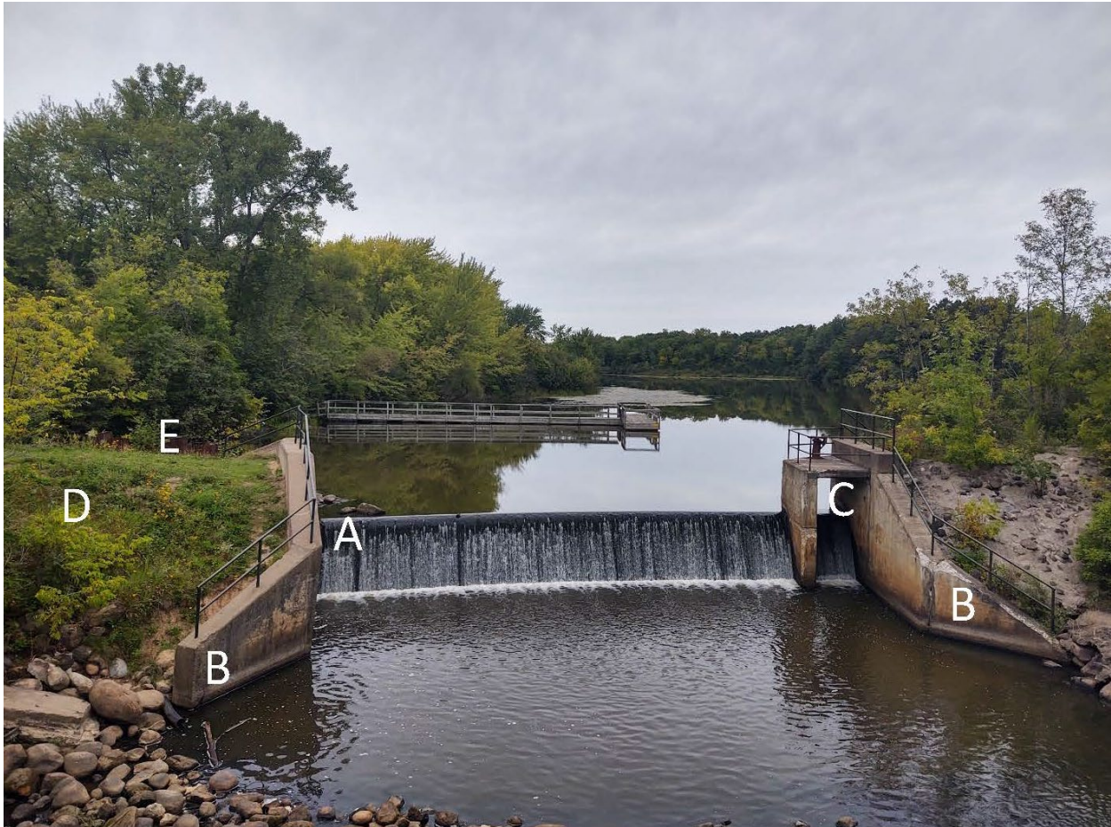
Figure 1-1. Grindstone Dam located on the Grindstone River in Hinckley, Minnesota. The Grindstone River is in the foreground of the picture, the Grindstone Reservoir is located behind the dam. Labels: A. Concrete spillway; B. Left & Right Abutments; C. Sluice gate. ; D. Embankment, and E. Sheetpiling.
