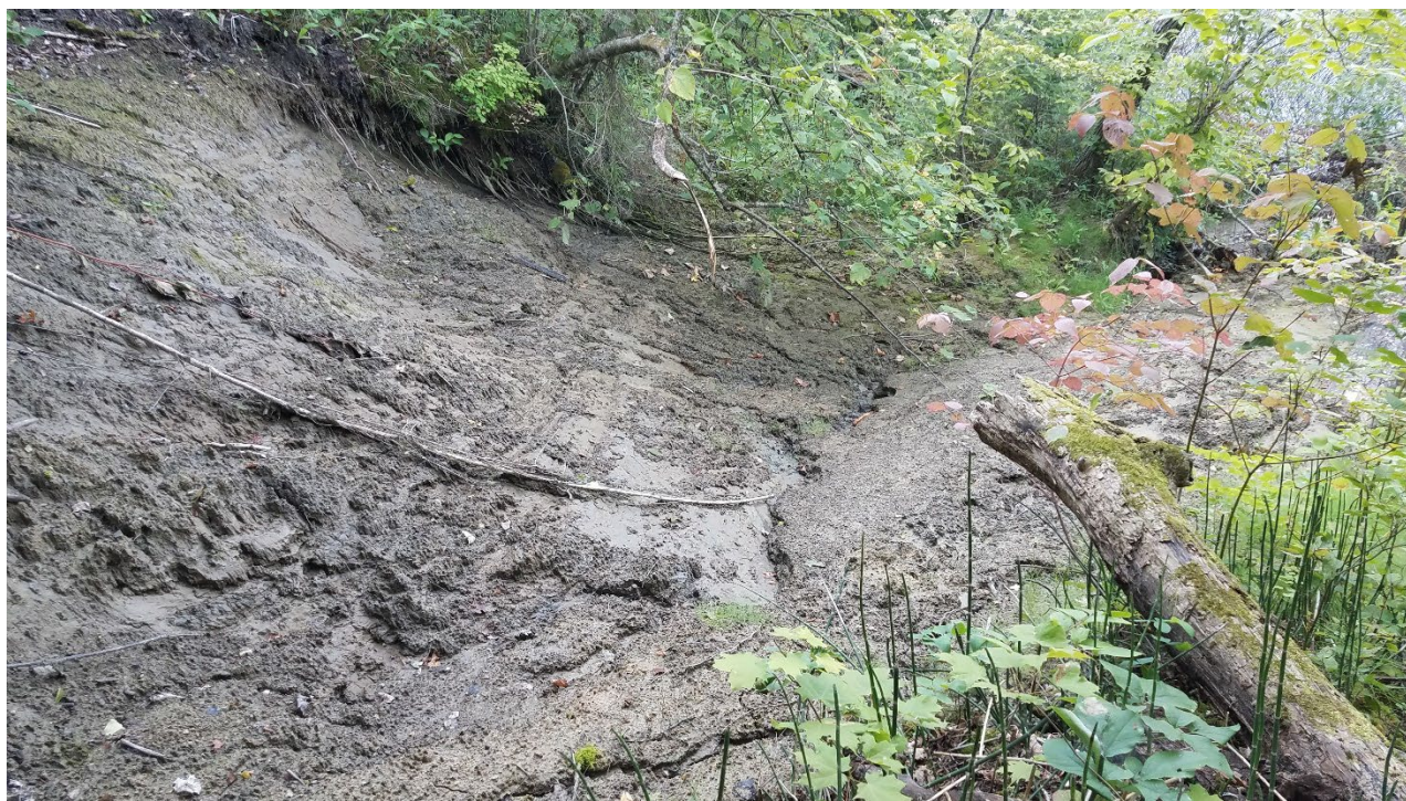
Photo 37 Bottom of sluffing slope pre-project 2019. Adjacent lakeshore is visible in the upper right.
