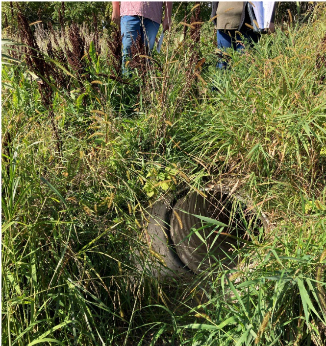
Photo 14 Culvert outlet into west side of wetland basin. Seeded and ruderal vegetation is well established from the outlet to the wetland pond.
