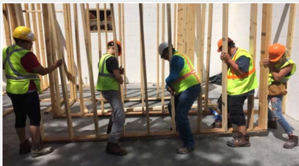
Stormi, John, Jason (Construction Coordinator), Shane, and Nita set interior walls in the basement of a ground-up building project.
