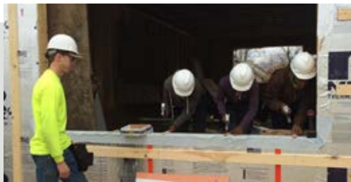
Tree Trust YouthBuild construct a new Urban Homeworks house in north Minneapolis.
