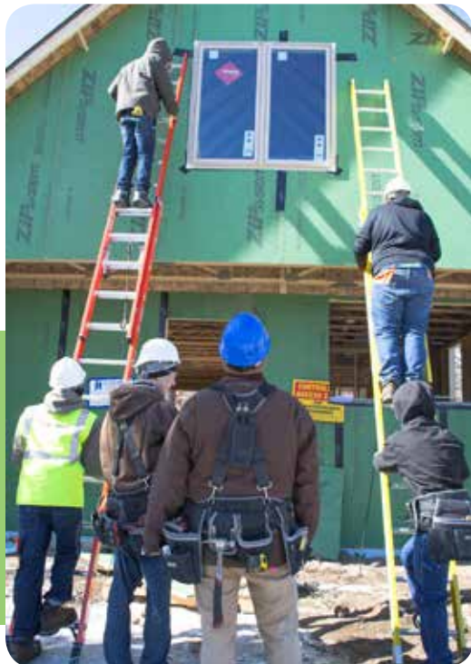
Green home being built by the Tree Trust Youthbuild crew in north side of Minneapolis.
