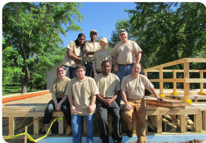
Clay, Jaden, Travonta, Mohamed, Anas, and Samantha take a break after construction of the wooden headers with instructors Dave Masters and Bill Garceau.
