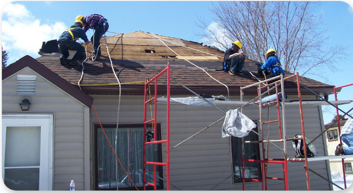
Eric, Levi, Kyle, and Miranda reroofing a Bi-CAP transitional house in Blackduck.
