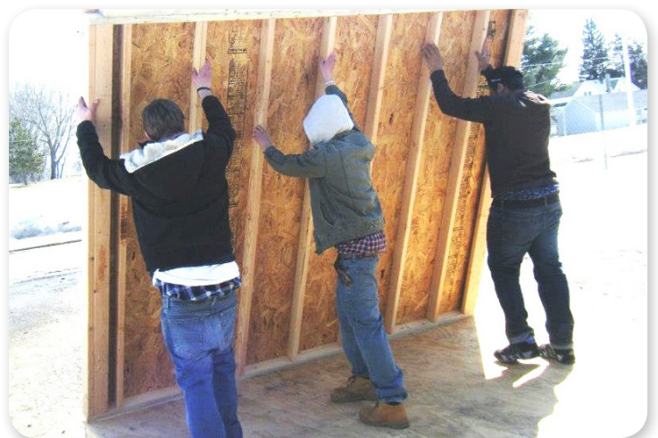
Dustin, Mckenna, and Derrick lift up the side wall during a storage shed framing project in Wabasha.
