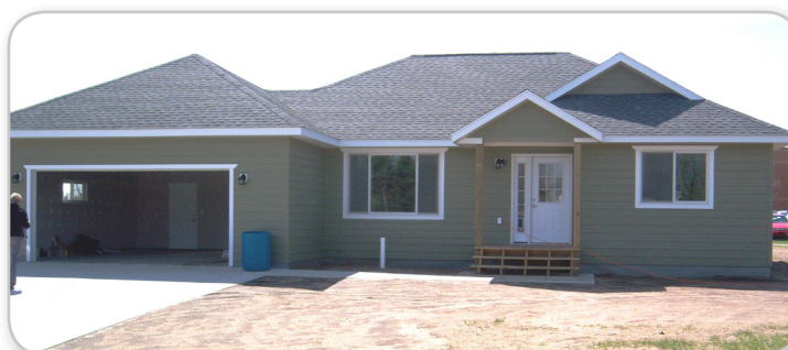
Youthbuilders built a single family home for a low income family with the Housing Authority and the city of Perham.
