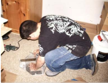
Thomas measuring strips for finish work on the Robie house in St. Paul.
