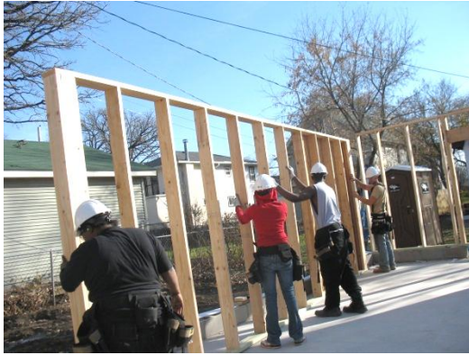
Tomaine and Monica frame the exterior walls of a north Minneapolis garage.
