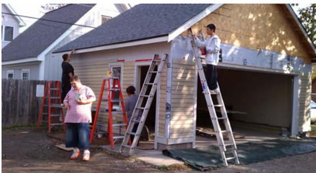
Youthbuilders build a new garage on Douglas Street on St. Paul's eastside.
