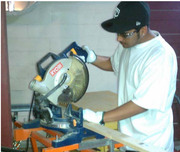
Isaiah measures and cuts wood studs for house renovation project on Hawthorne Ave on St. Paul's eastside.
