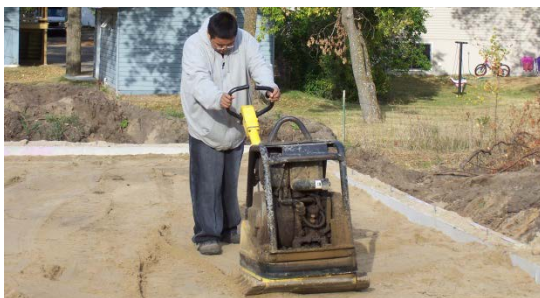
Eldon operates a packer to prepare the foundation for a home in Bemidji.
