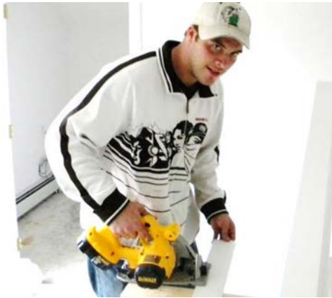
Mike enjoys using the cordless saw during his renovation work at a house being built in Eveleth.
