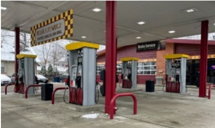
Newly installed E2- compatible fuel dispensers at Nelson Auto World in Minneapolis, Minn.
