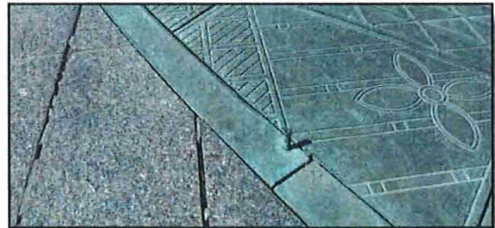
Metal pin is a trip hazard.
