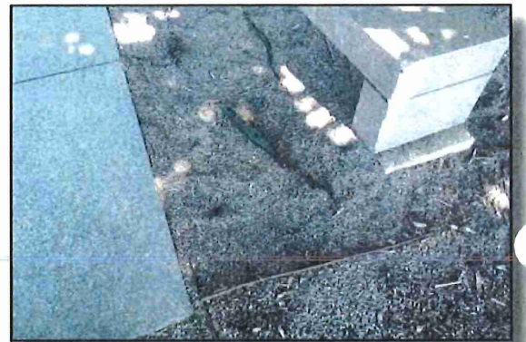
Landscape fabric under pea gravel is a trip hazard.
