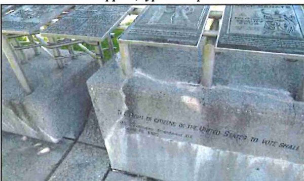
Wall has cracked and needs granite replacement for inscription.
