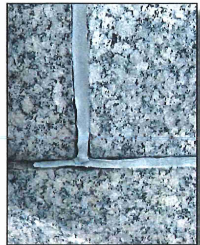
Joints need to be reworked.
