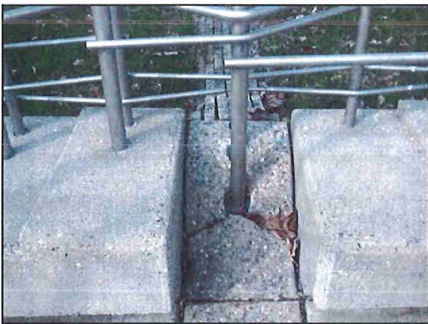
Failed concrete support, typical at post wall.
