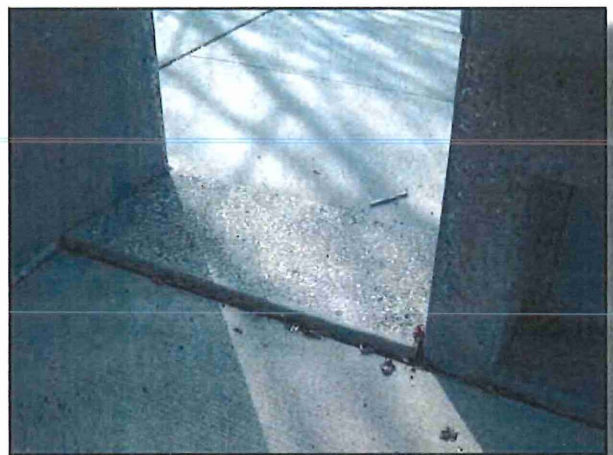
Trip hazard at adjacent podium.
