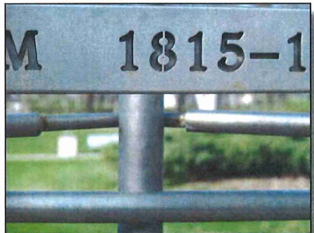
Rusting surface needs protective coating.
