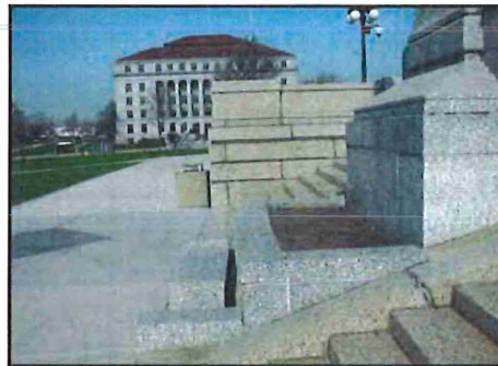
Stone needs to be reset.
