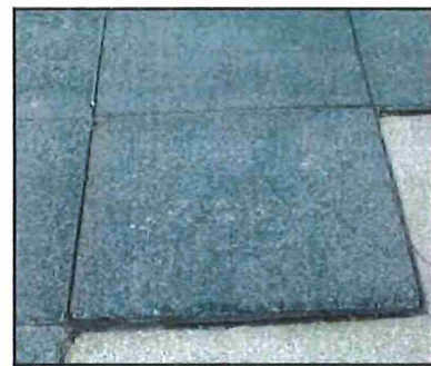
Paving trip hazard needs correction.
