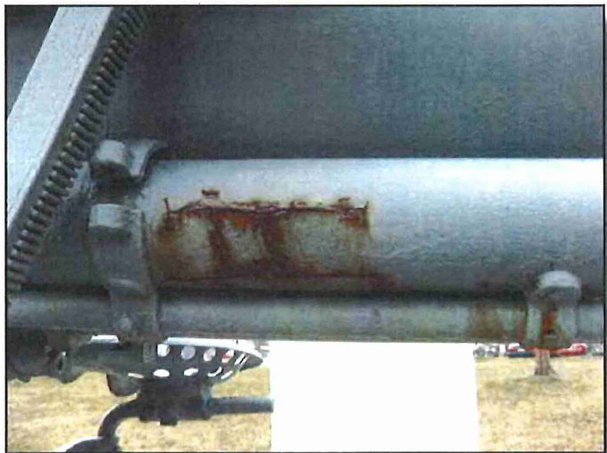
Repair rusted areas and repaint entirely.
