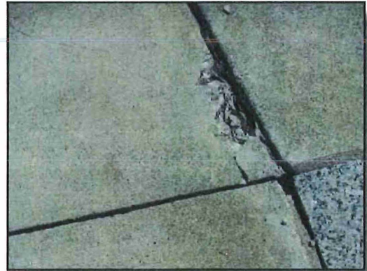
Sidewalk and pavers need replacement.
