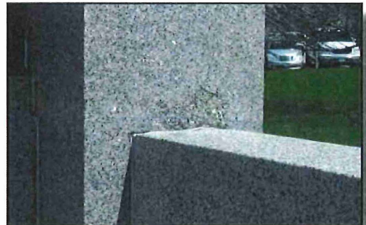
Joint needs work to prevent additional spalling of stone.
