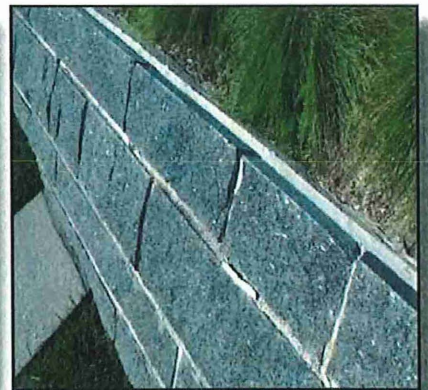
Wall needs tuckpointing.
