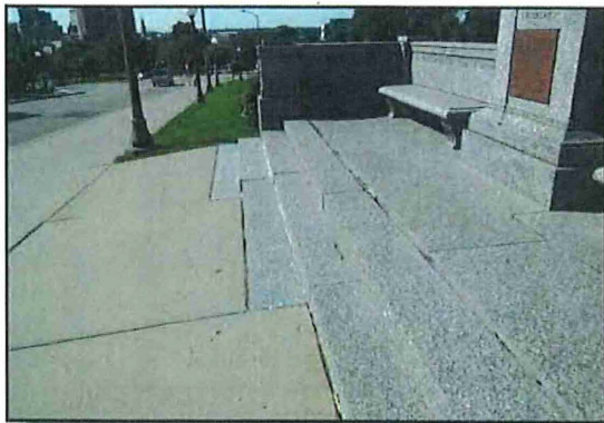
Only stairs need resetting.
