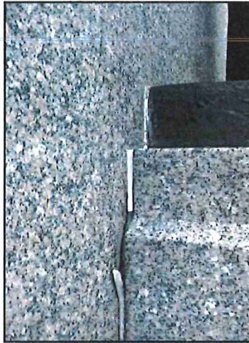
Joints need to be reworked.
