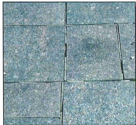
Granite pavers need to be reset to eliminate trip hazard.
