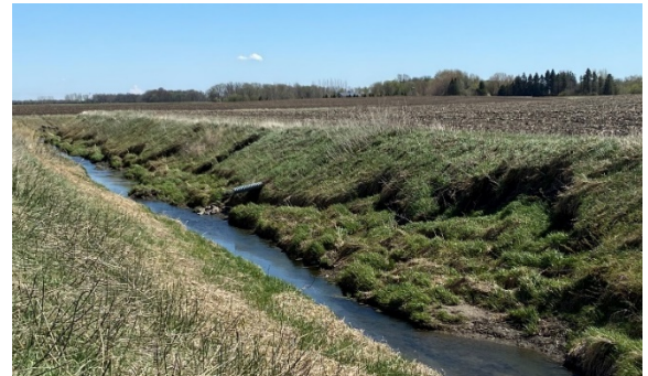
Figure 12: Slumping of stream/ditch banks just north of SMC1 monitoring site, 2021
