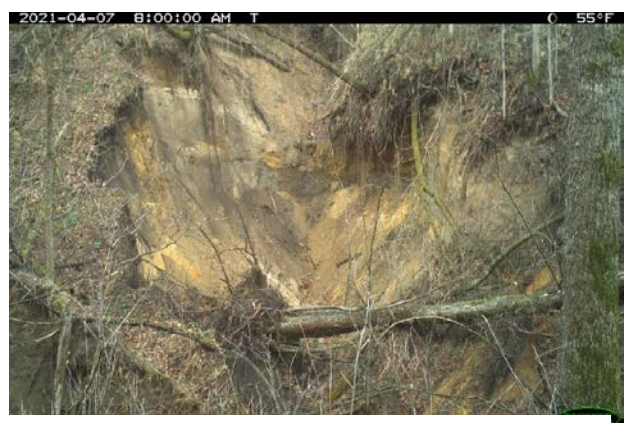
Figure 11: Ravine erosion captured from field camera in Seven Mile Creek Park
