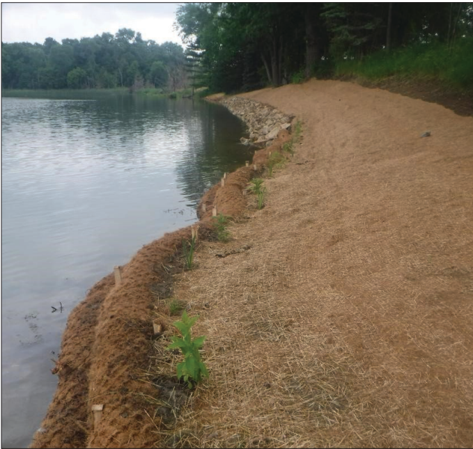
Shoreline stabilization projects by the Scott Soil & Water Conservation District helped to improve water quality and reduce phosphorus in McMahon Lake.
