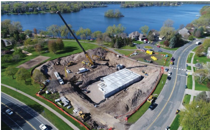
Burnsville built an underground stormwater treatment system to reduce contaminants in water flowing into Keller Lake. Crystal Lake is in the background.
