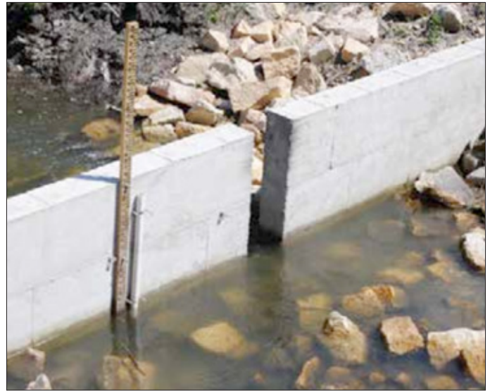
Low flow in the Ditch 57 Rate Control Weir – Blue Earth County, MN (Source: ISG)
