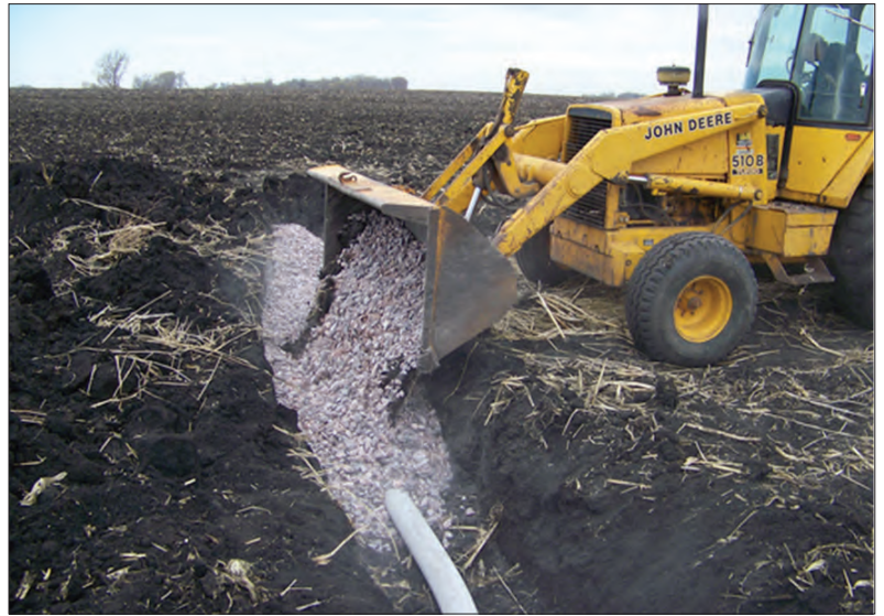
Rock tile installation, a successful BMP during the High Island Creek TMDL Project for fecal coliform
