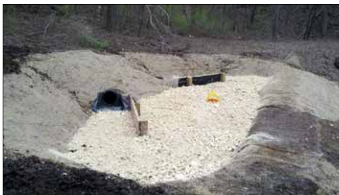
Installation of the spent lime test cell on the NW corner of Larpenteur Avenue and Prosperity Road in Maplewood, Minnesota.
