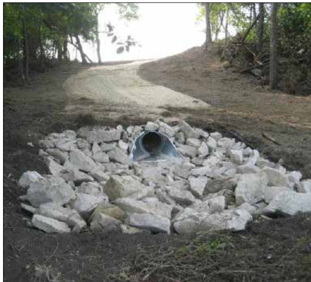
This outlet grade stabilization structure project was located in NW ¼ of Section 32 of South Bend Township in Blue Earth County, Minnesota
