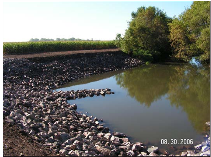
This picture shows a bank on the Cottonwood River after the implementation of bank stabilization including stream barbs to keep the river from heavy erosion on the outside bank. The project is on the Cottonwood River in Gales Township, Redwood County.
