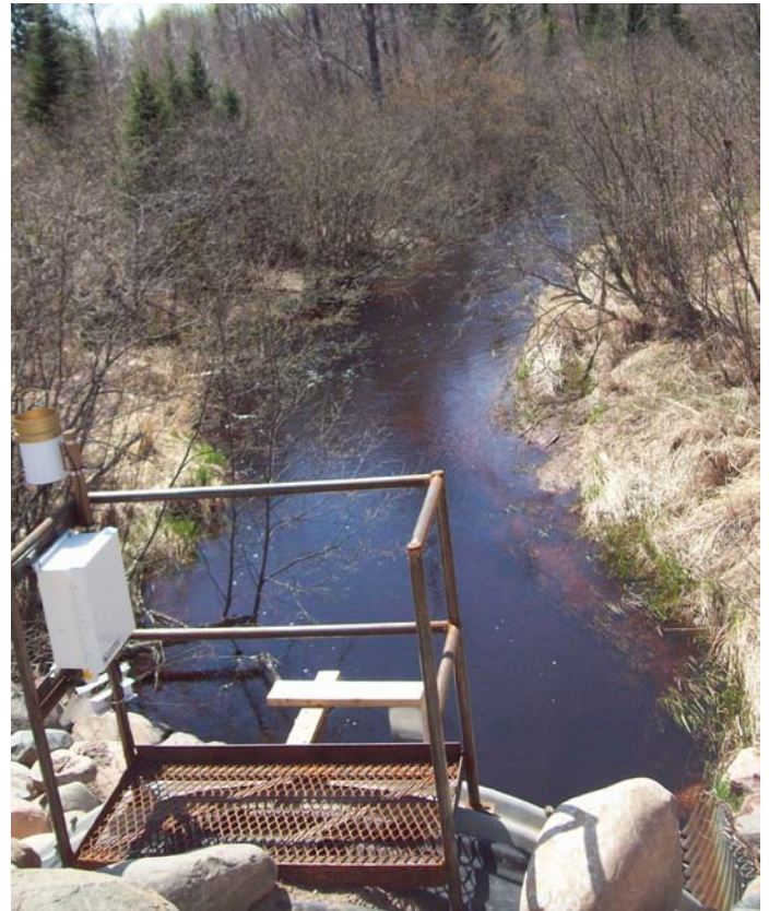
Blackhoof River Monitoring Station: The SWCD worked with County Transportation Department to construct a safe walkout structure for a new stream-monitoring site as part of the TMDL load monitoring for the Nemadji River. 9 new monitoring sites were developed for this project.
