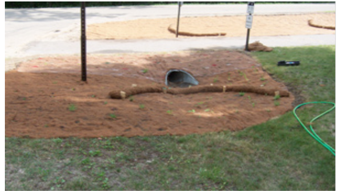
Installing erosion control measures at the rain garden site between Crest Ridge Road and the Lake Koronis Recreational Trail.
