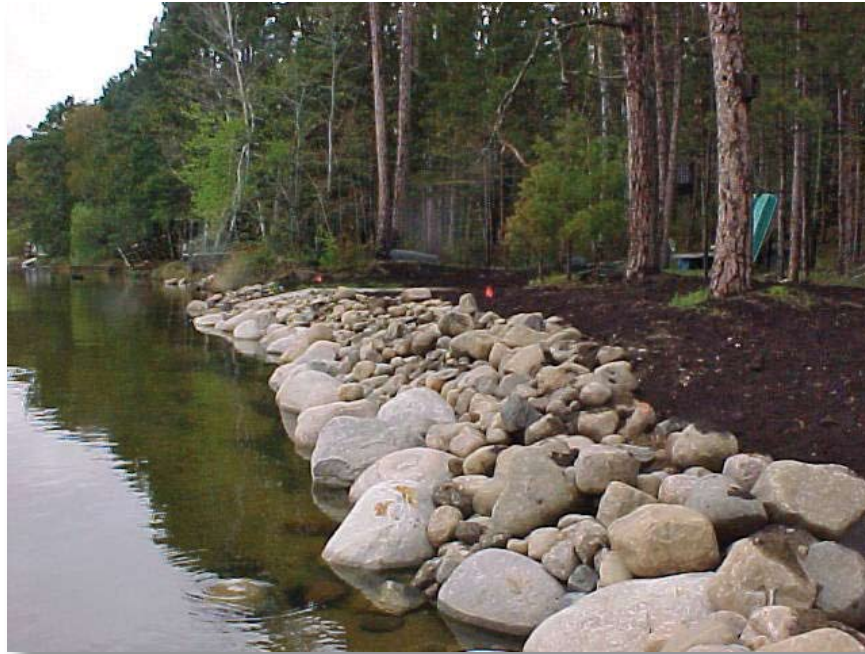
Riprap was installed to prevent soil erosion on 800 feet of Lake Minnewawa's shoreline.
