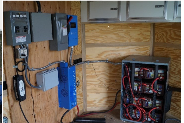
Solar Trailer Equipment with Original Lead-Acid Batteries
