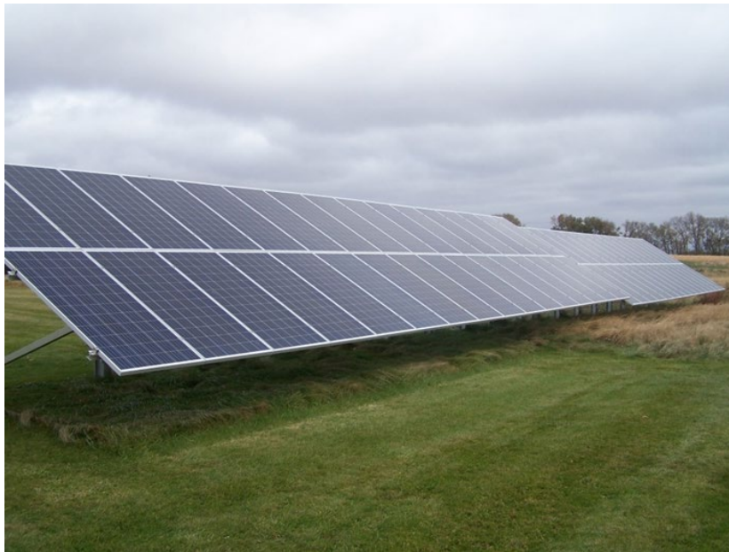
Figure 3. Solar panels (20 kW) installed at the WCROC used to power the sow cooling system
