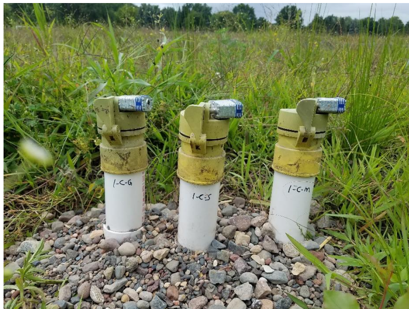
Figure 2-4: Photograph of Three Sampling Ports of a Monitoring Array Used to Collect Treated Water from Gravel (G), Sand (S), and Sorption Media (M) Layers in VFB Cell 1
