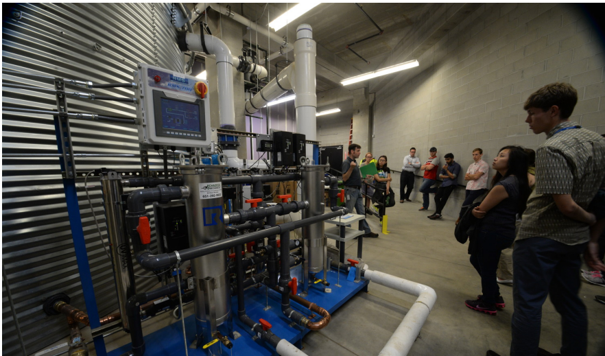
Figure 15. Stormwater reuse is showcased on tours of the cistern that holds rainwater captured from the roof of Metro Transit's Green Line Operations and Maintenance Facility, for use at CHS Field.
