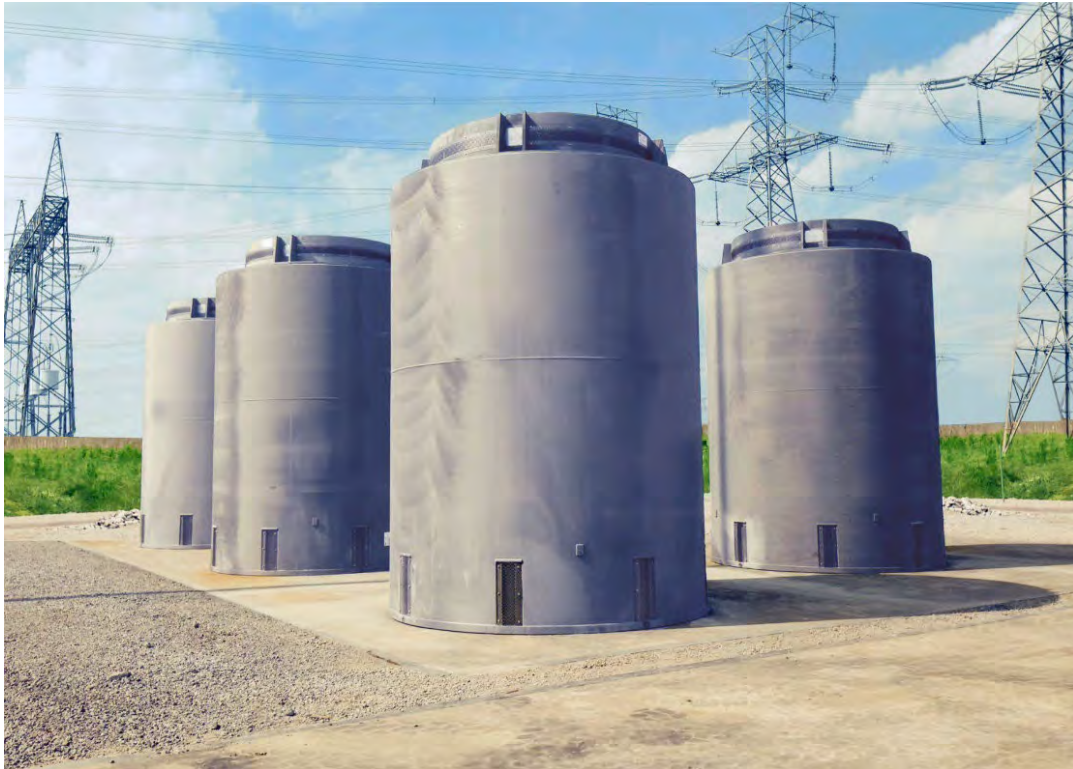
Figure 4. Vertical Canisters in Concrete Overpack
