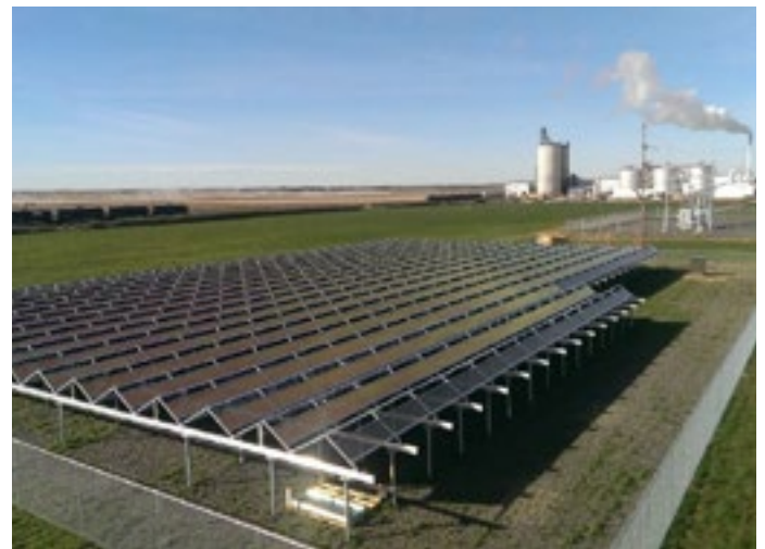
Redwood Electric Cooperative's 134kw community solar array near Lambertton. Visible in the background is Highwater Ethanol.
