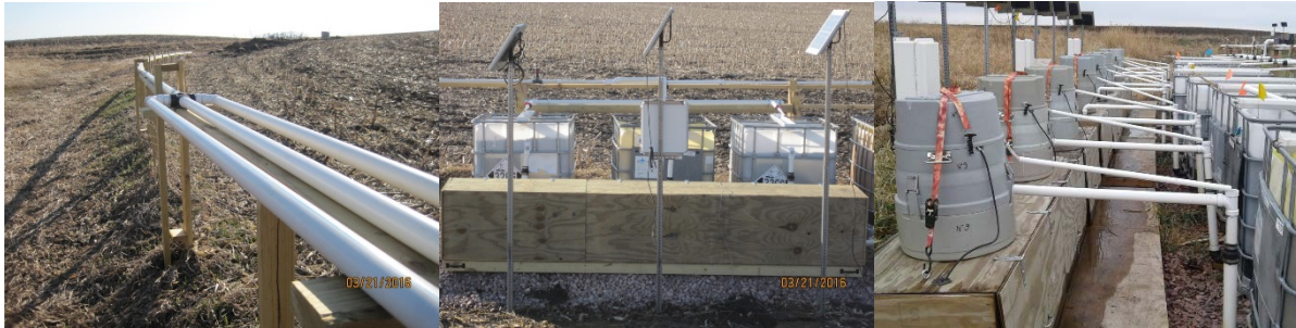
Figure 4.4. From the left: three-way subsurface drain flow splitter to distribute water from the subsurface drain outlet to the bioreactors; block of three bioreactors with a set of three solar panels, one paddle wheel, and a datalogger in the white enclosure; portable samplers for collecting bioreactor discharge for water quality component analysis.
