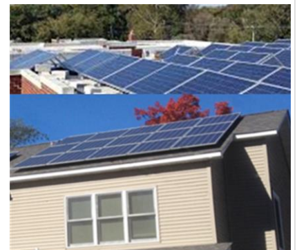
Figure 13. Solar PV systems
