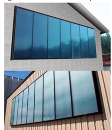
Figure 14. Solar thermal systems
