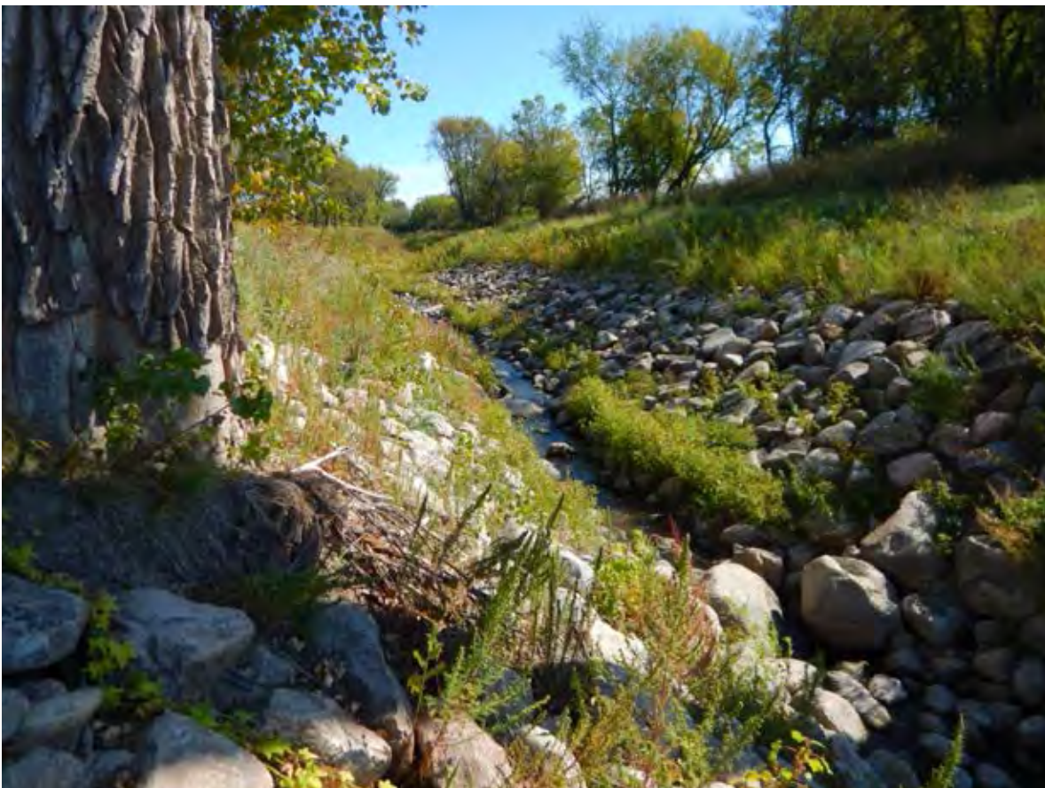
SR Photo 36: V Channel immediately upstream of confluence with the Red River. Note scour at base of cottonwood tree at top of slope.
