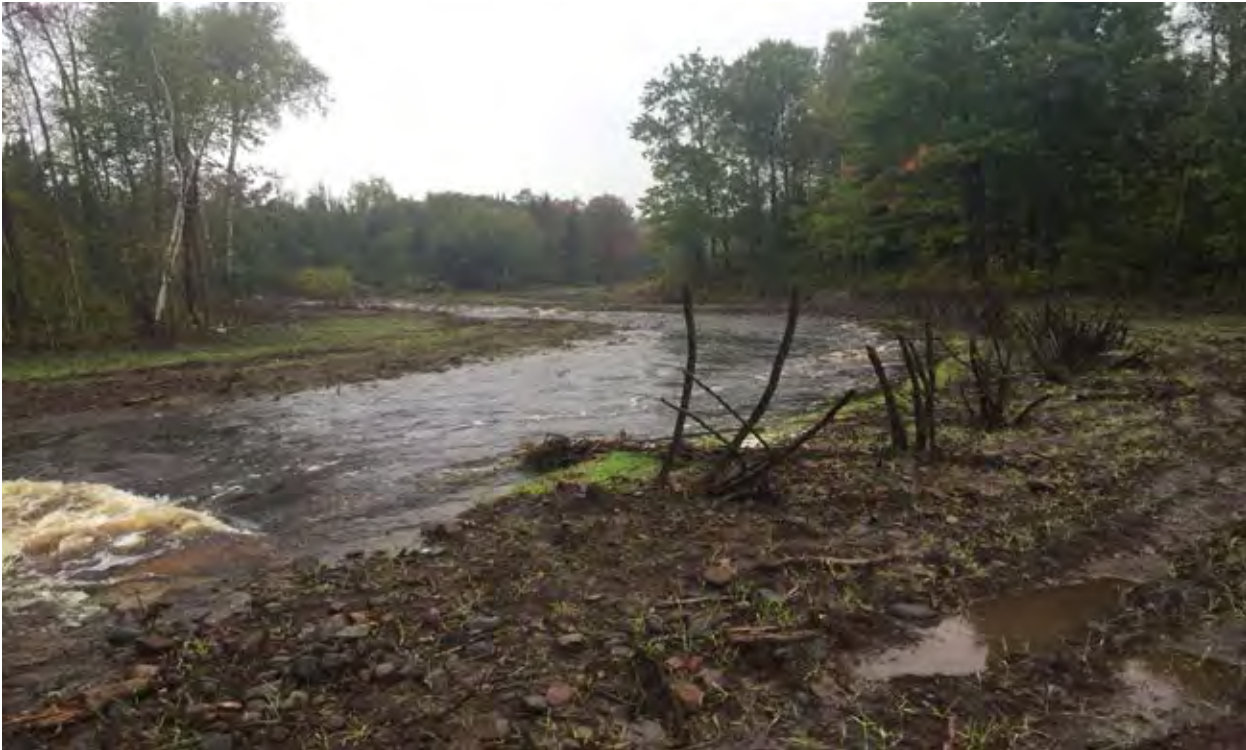
Figure 5 - Representative image of project elements: Toe Wood (right) with willow harvested mats above and Log J Hook with Rootwad downstream (left).
