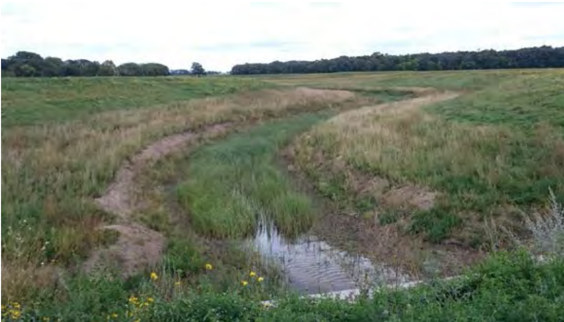
SR Photo 8: Constructed Channel looking east from 470th Avenue NW. Seeded upland, unseeded channel.
