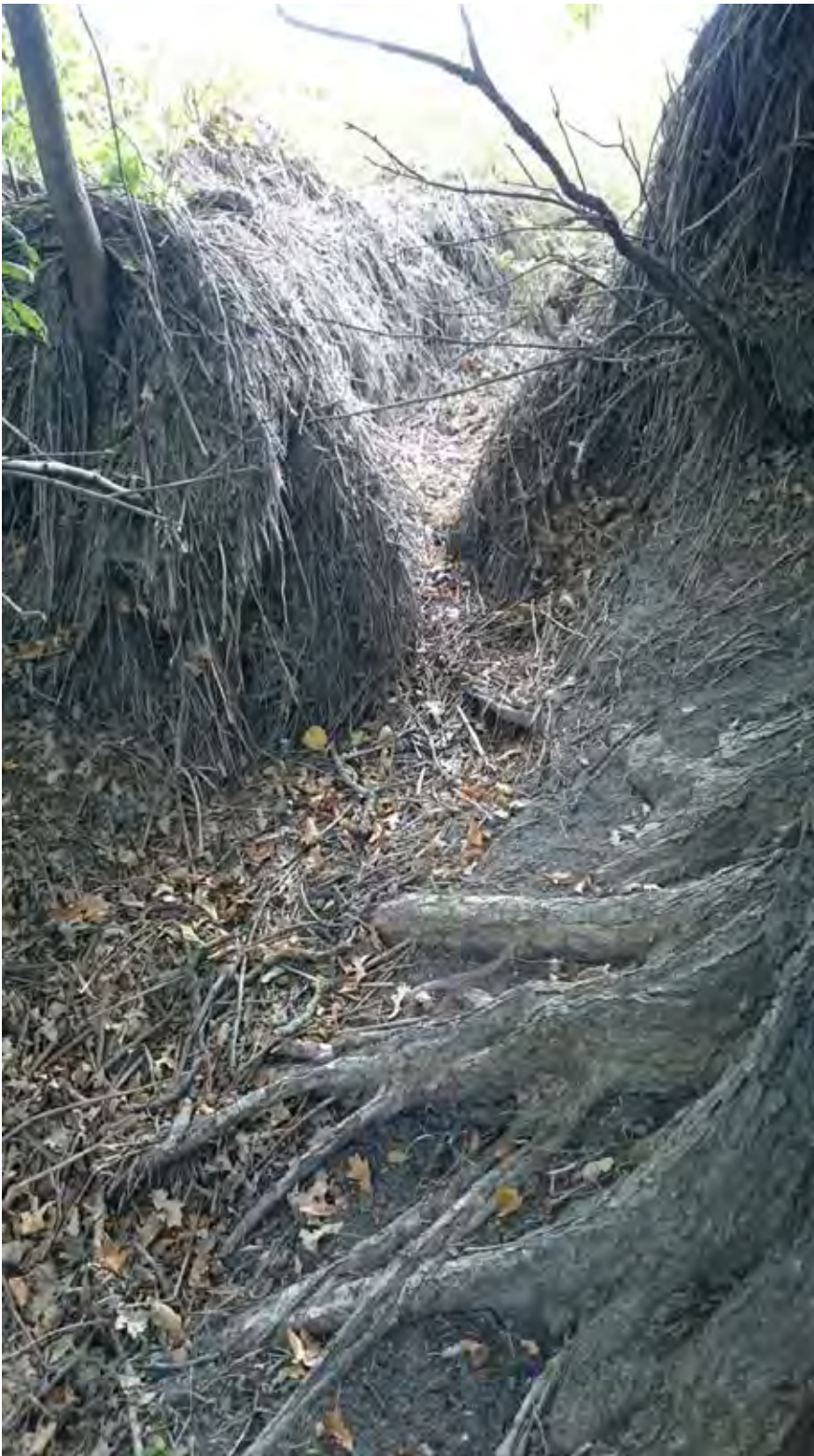
SR Photo 28: Gully above construction area in wooded area. Likely predates project as it is above existing exposed roots.
