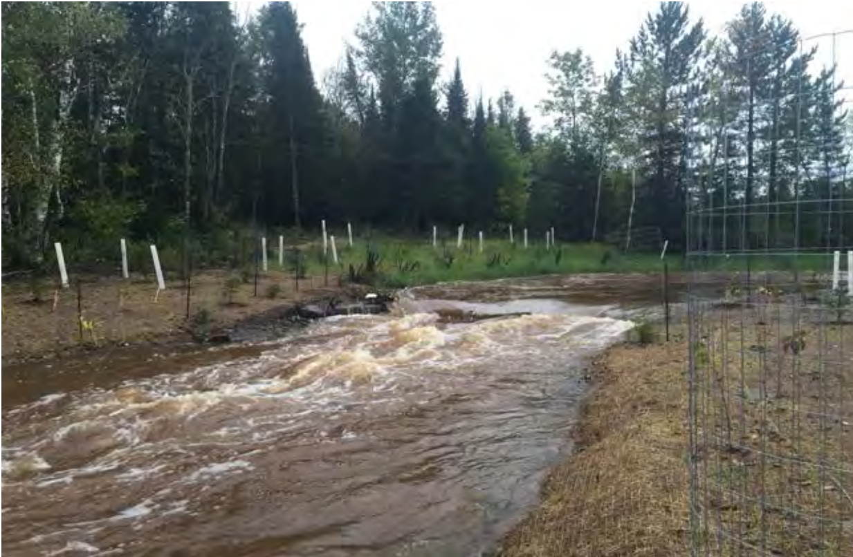
Figure 3 - Representative image of stabilization. Note the grade control structure (center images) was a project add-on (understood to have been requested and/or funded separately by Minnesota Trout Unlimited).
