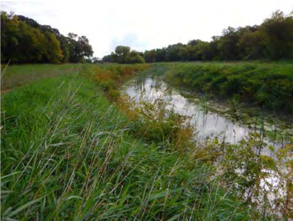
SR Photo 2: Vegetated slopes in upper project area immediately downstream of Diversion Structure.
