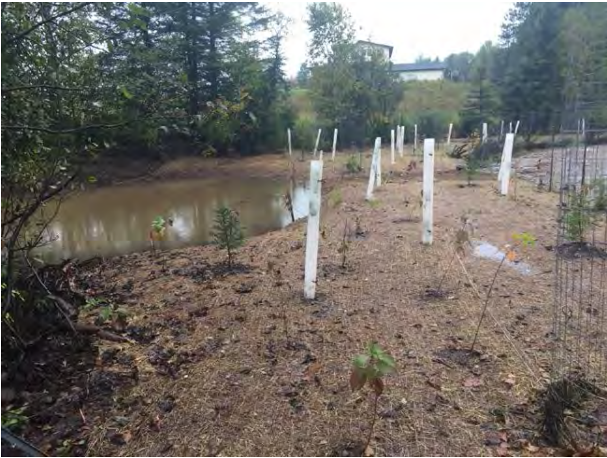
Figure 5 - A constructed offline "wildlife pond" (left side of image), a minor project change, was a product of balancing cut & fill.
