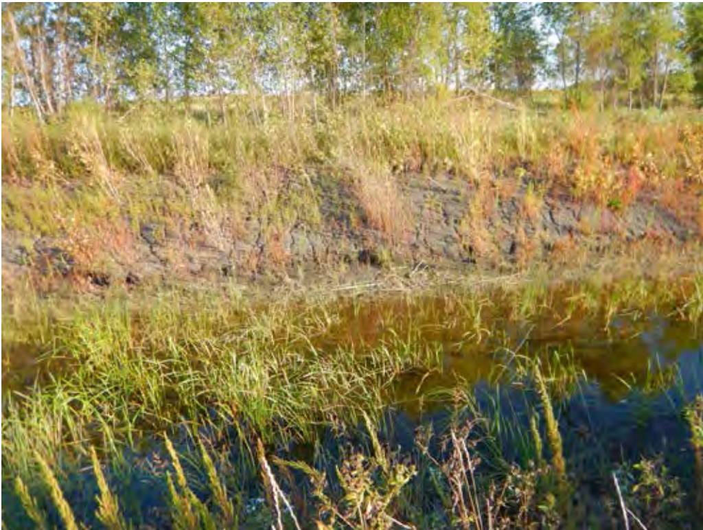
SR Photo 13: Unseeded slope at excavated channel.
