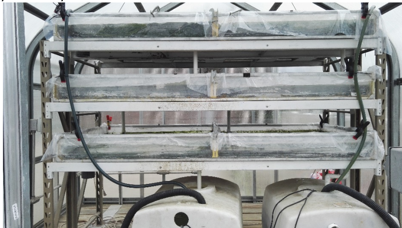
Fig.1 Two PBRs system at the Metro Wastewater Treatment Plant.
