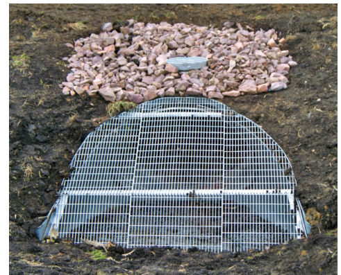
A culvert screen installed in southwestern Minnesota to prevent invasive carp moving from the Missouri River water shed into the Des Moines River watershed during high water events.
