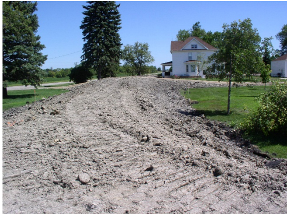
Figure 19. Example of ring dike constructed to prevent contamination of flood water during flood events.
