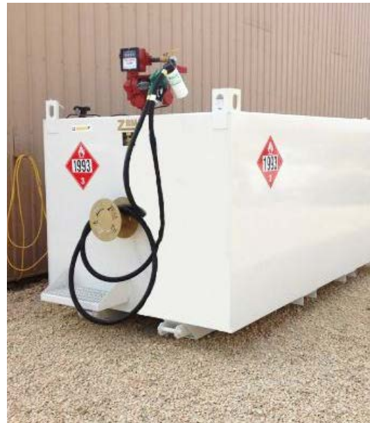
Figure 31. Example of a double wall containment tank funded by the AgBMP Loan Program
