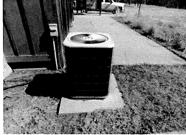
Air conditioner is also 11 years old SEER 10 unit.
