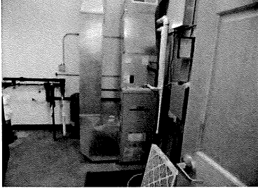
Existing furnace is an 11 year old 92% efficient furnace. The supply air runs through the attic.
