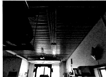
Typical 8' light fixtures in shop.
