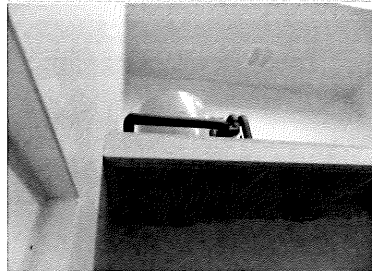
Hot water heater for shop.
