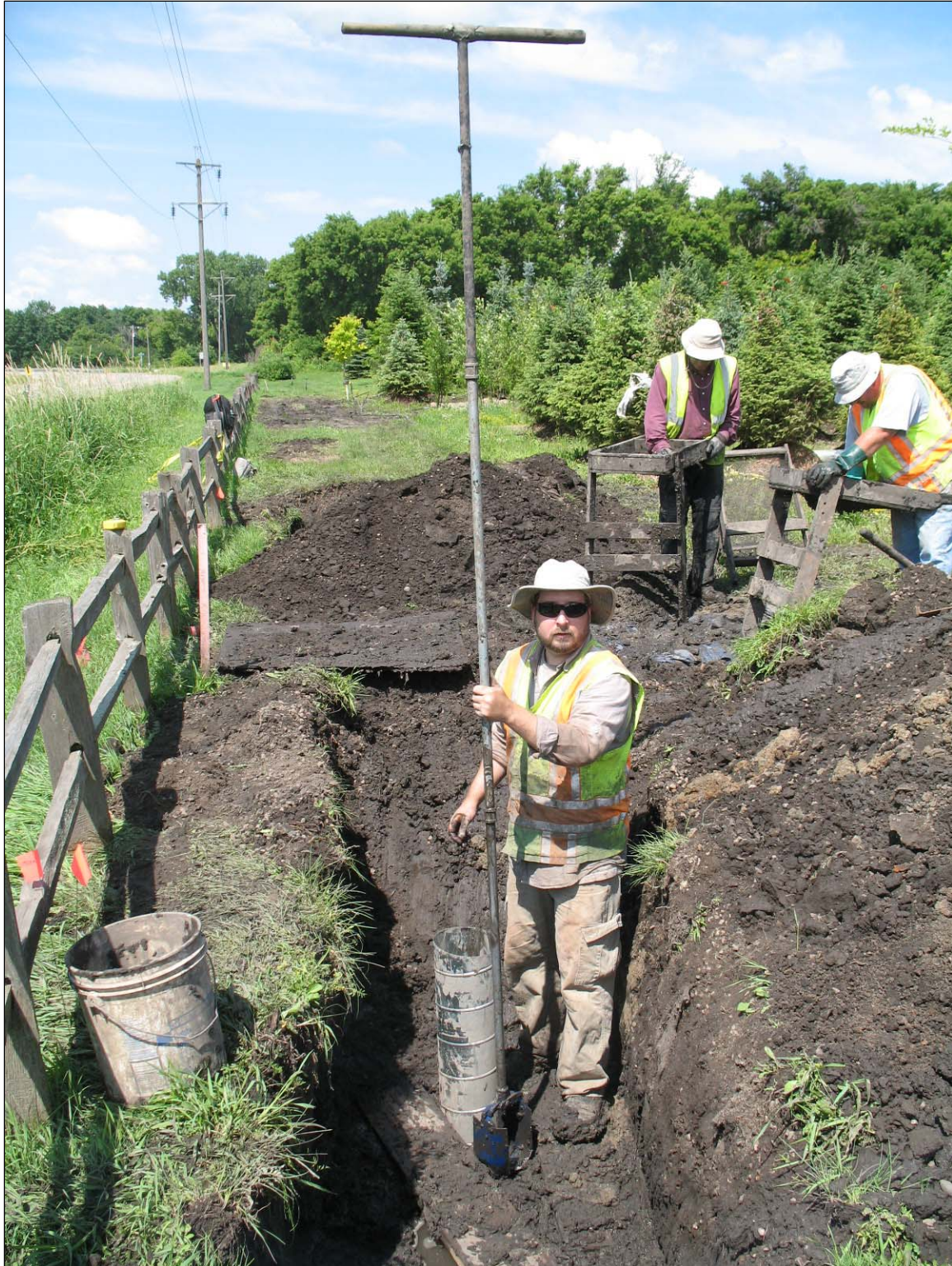
Figure 29. Site 21CR155 Photo of Auger Testing in Backhoe Trench at Brookside Garden Center on North Side of CSAH 61 at ST 31G, Facing West.
