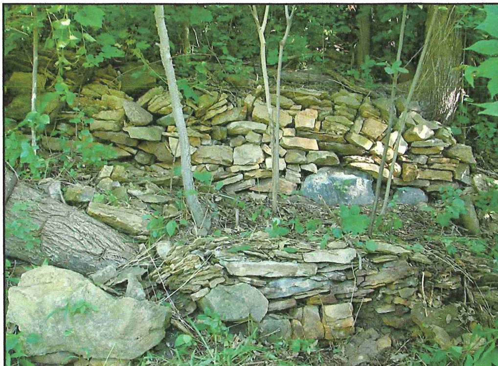
FIGURE 20. SHORT DRY-LAID RETAINING WALL IN FOREGROUND WITH A SECTION OF THE LONG RETAINING WALL IN THE BACKGROUND, VIEW TO NORTH
