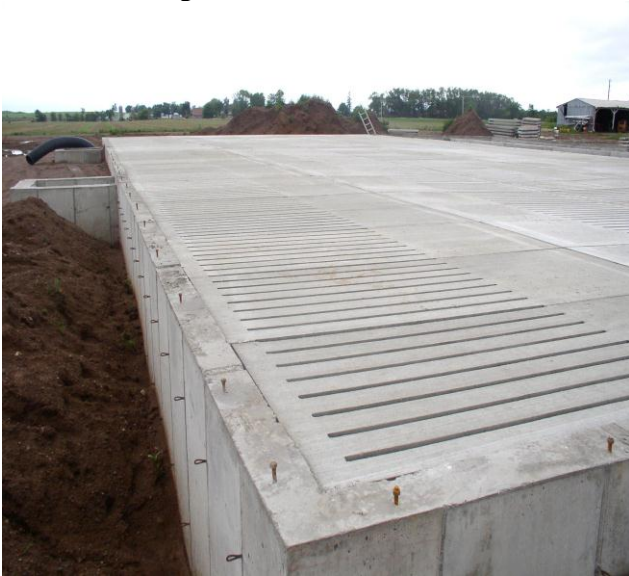
2. Figure 5. Typical concrete slatted floor manure storage basin
