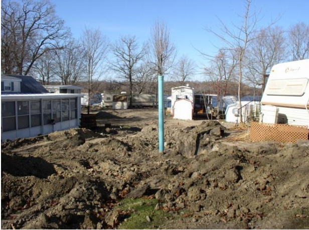
Figure 43. Construction of collection system in park at Happy's Landing Association, Douglas County, MN.
