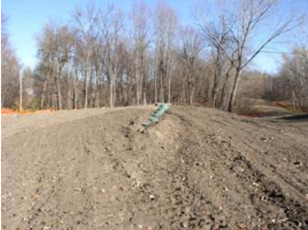
Figure 18. One of two treatment drainfields at Happy's Landing Association, Douglas County, MN.
