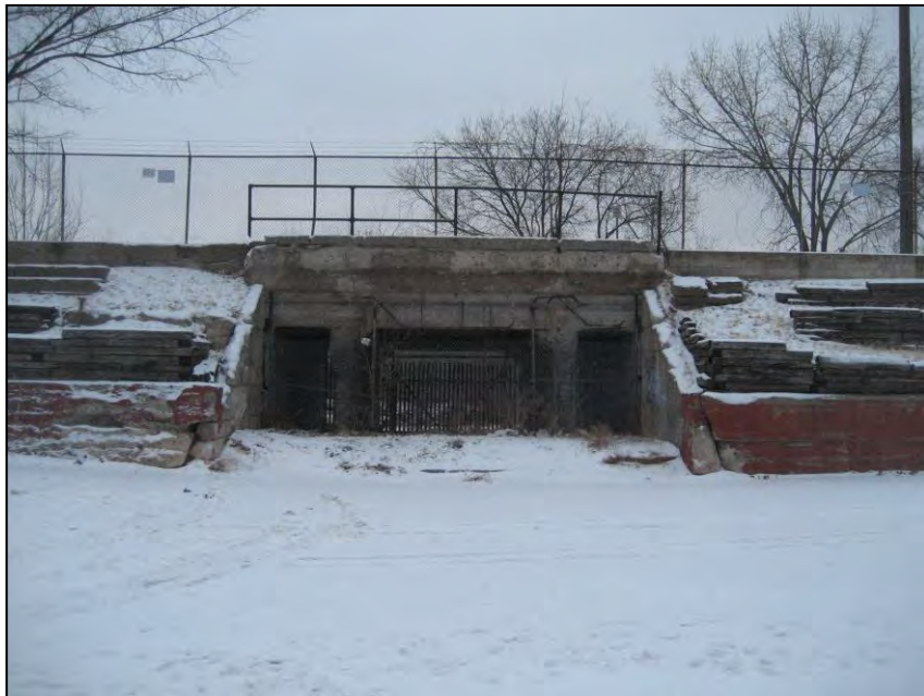
Below: Tunnel below Twenty-ninth Street at the north end of the property. The former railroad corridor is on the other side of the tunnel. View to north.
