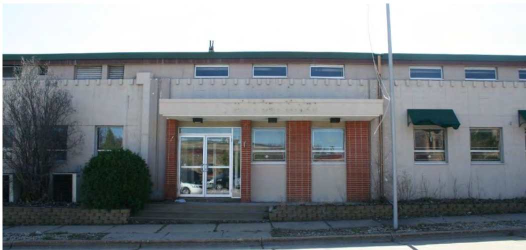
Figure 44. Primary entry of the warehouse on the northwest (front) façade, view facing southeast.
