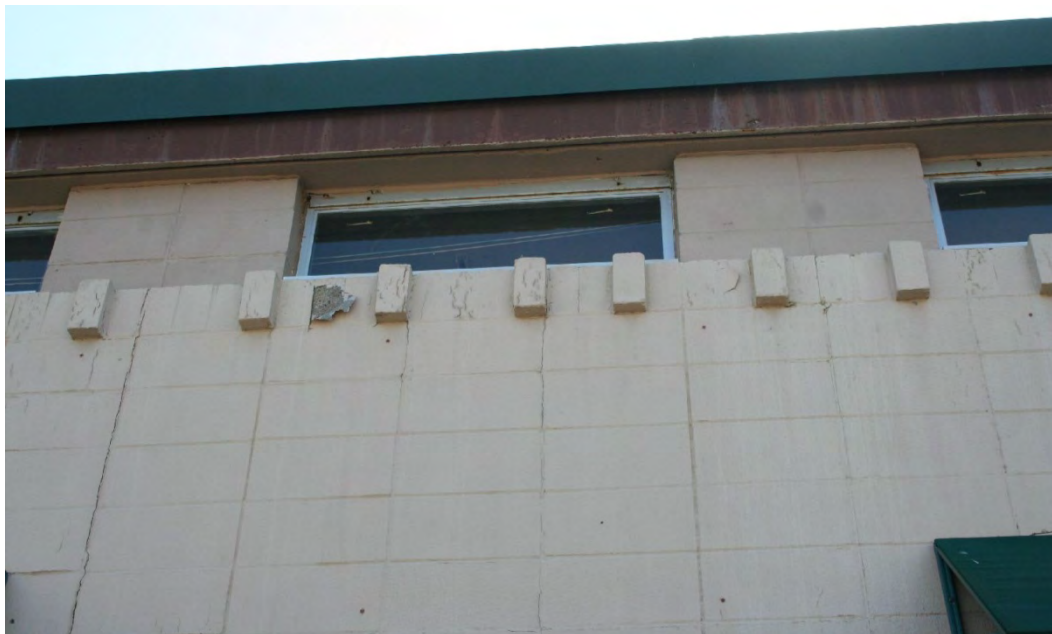
Figure 43. Detail of concrete dentil work that encircles the warehouse, view facing southeast.
