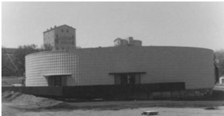
Figure 84. East side of the Motor Travel Services Building under construction (Image from St. Louis Park Historical Society website, www.slphistory.org ).
