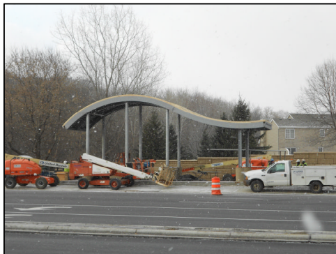
Figure 11: (left) Construction of new walk-up station at 140 th Street. (right) New Red Line Bus Rapid Transit Vehicle unveiled on December 10, 2012.
