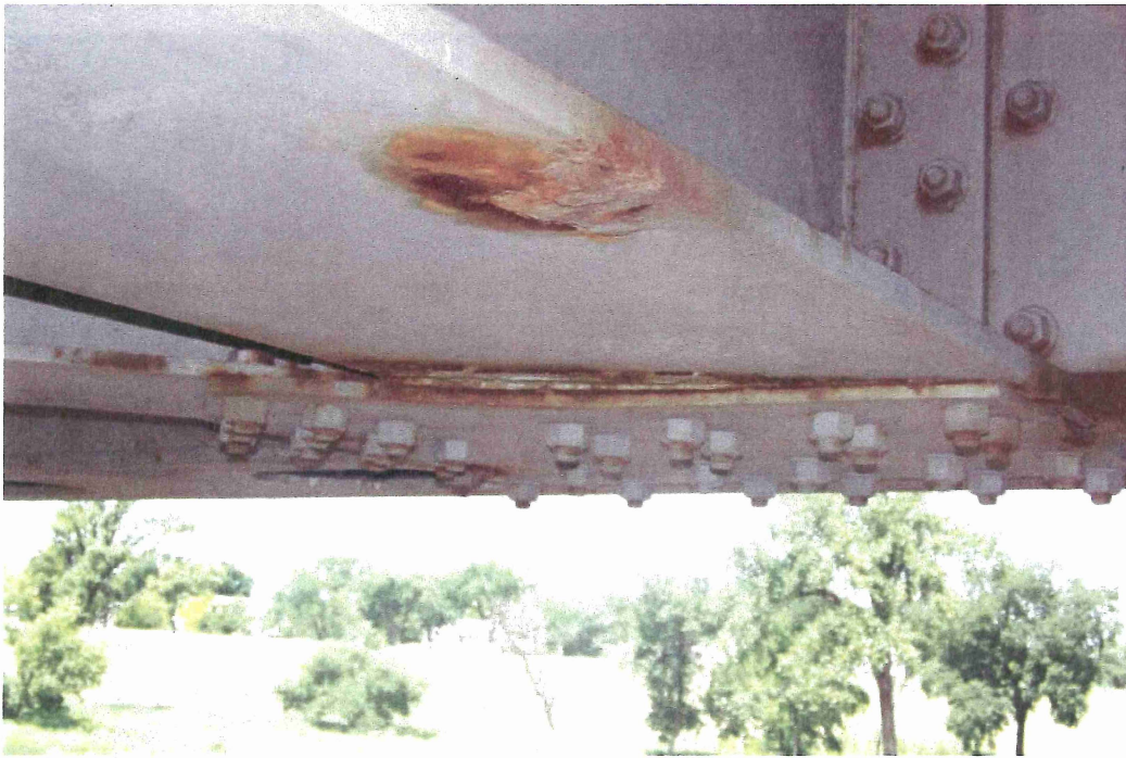
Photo 25 – East Truss Span (Span 7), north truss at panel point L3'. Note pack rust (3/8") between lower horizontal connection plate to bottom flange of floorbeam. This condition is randomly found throughout the truss spans.
