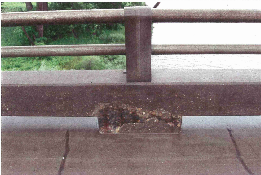
Photo 5 – Span 7, concrete spall in parapet post with exposed rebar, looking south. Cracking of concrete and insufficient concrete cover has caused spalls to develop at random location along each parapet.
