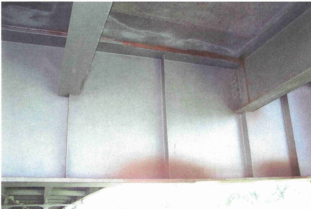
Photo 24 – Typical pumping of deck above floorbeams in truss spans. Pumping of deck is most evident at either end of floorbeam and at mid span.
