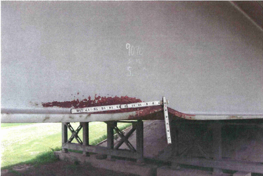
Photo 17 – Span 12, south fascia, impact damage to bottom flange. Bottom flange has been bent upward 2". Looking northeast.
