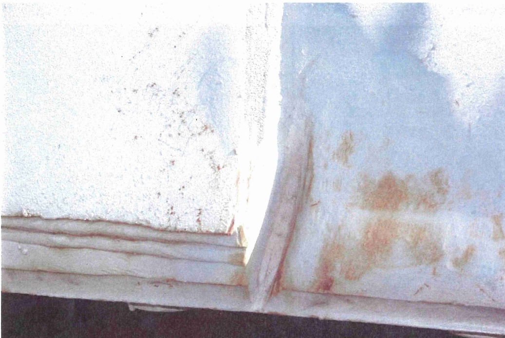
Photo 18 – West span, south truss, panel point L0. Location where crack was previous removed by grinding and caulked. Note visible signs of new cracks. Looking north.
