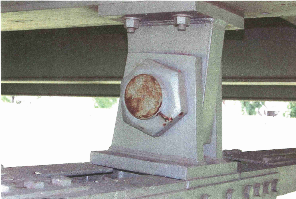
Photo 19 – Typical fixed support over Bents 2 to 5, and 9 to 13. Photo taken at Bent 5, Stringer 6, missing cotter pin on south side.
