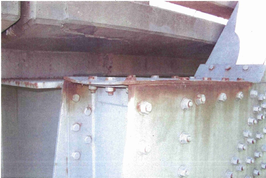
Photo 13 – North truss, west span, panel point L0'. Top batten plate has heavy pack rust between plates causing bending of the out portion of the plate. Looking southwest.
