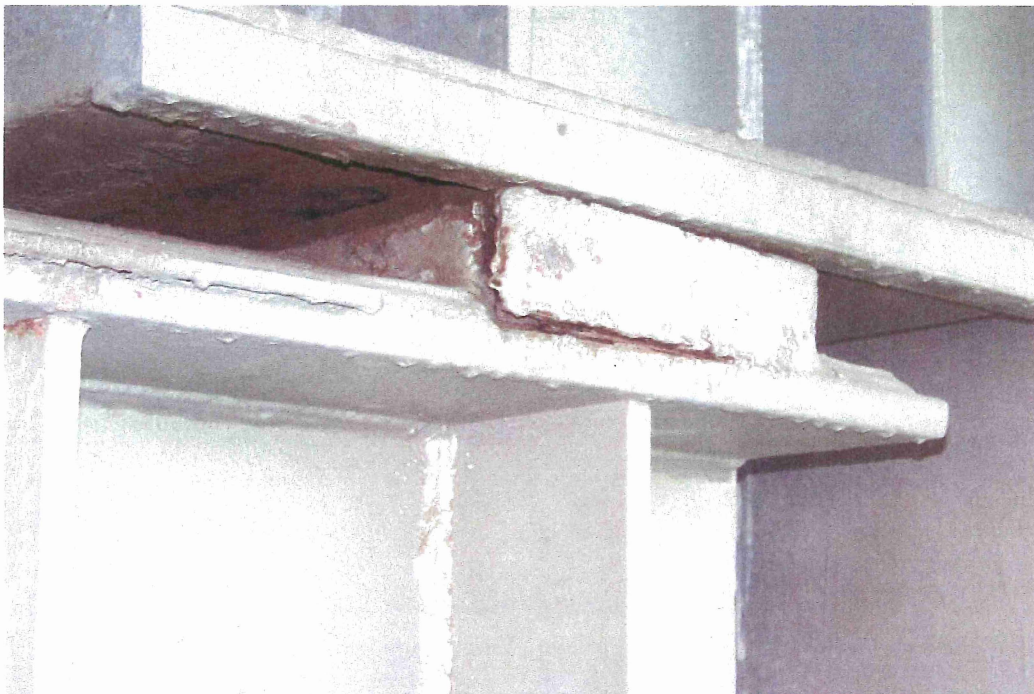
Photo 22 – Span 5, Stringer 1, cracked keeper plate weld.
