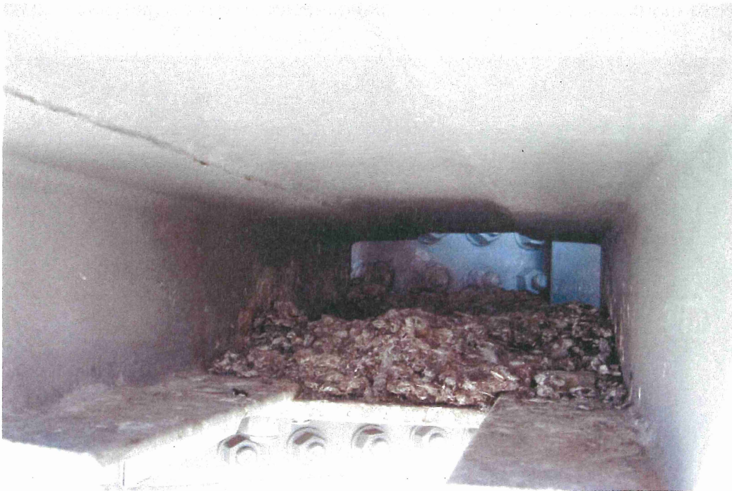
Photo 10 – At random locations inside the upper chord members, birds have nested. This nest is located in the lateral bracing adjacent to panel point U4'N.
