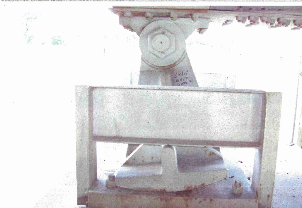
Photo 21 – Pier 6, north rocker bearing. Rocker bearing has rotated 8.4° to the west with an air temperature of 81 degrees. Looking north. Pintles are exposed.
