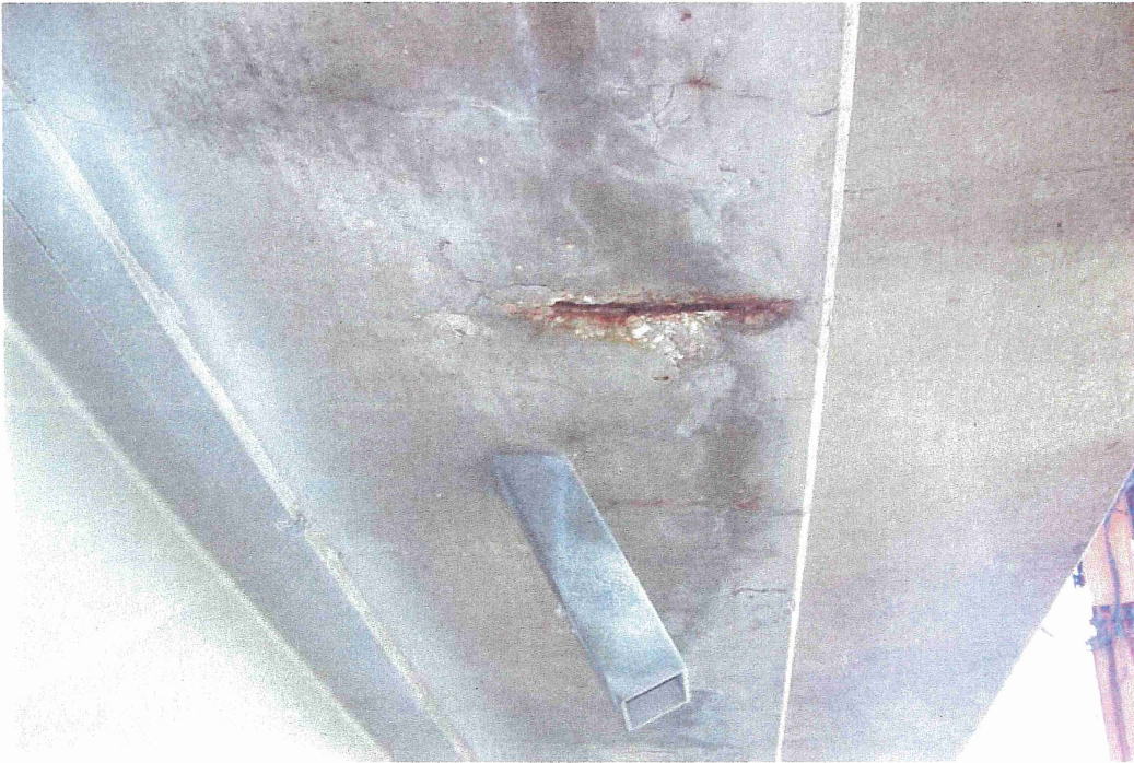
Photo 7 – East Truss Span (Span 7), random spall with exposed rebar in north soffit area. Note there is no downspout extension connected to deck outlet pipe. Looking up and west.
