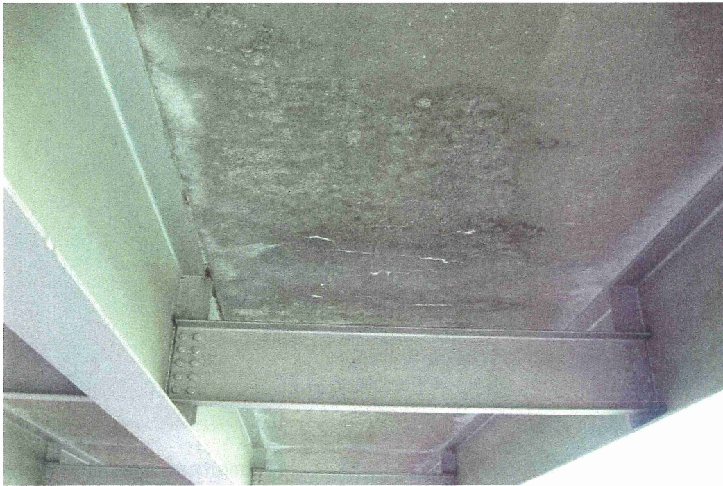
Photo 8 – Span 10, underside of deck slab between Stringers S1 and S2 exhibits an area of moisture contaminate deck, 5'x10'. Looking up and east.
