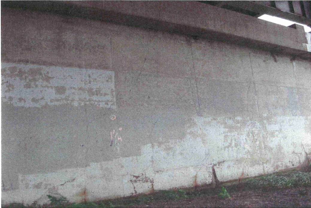
Photo 23 – Bent 6, east face, note 1/8" diagonal cracks in pier face. Similar cracks noted on west face however going in the opposite direction.
