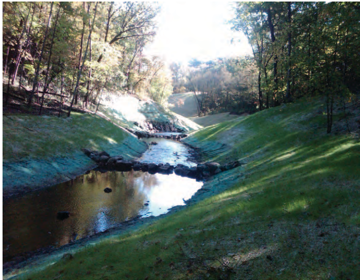
After: Scott WMO, working with the City of Savage and Scott SWCD, received $130,000 from the Clean Water Fund to install this BMP to stabilize the Utica Ravine, and help restore the Credit River.
