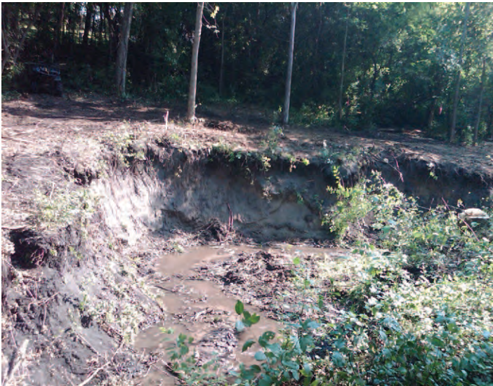
Before: Significant erosion from the Utica Ravine in the City of Savage was a large source of sediment to the turbidity-impaired Credit River.
