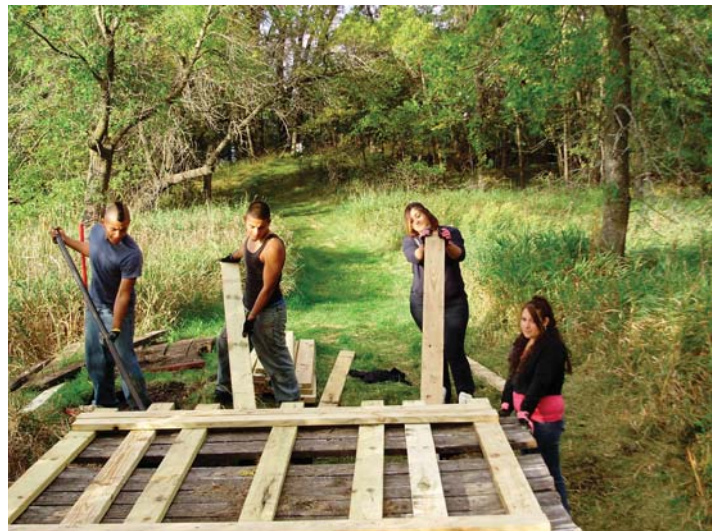
Photo above: Youthbuilders assist in the reconstruction of a dock for the Prairie Woods Environmental Learning Center in Spicer.
