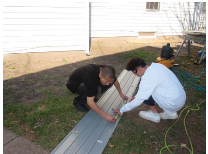
Photo above: Youthbuilders measure and install siding on a house in St. Paul.
