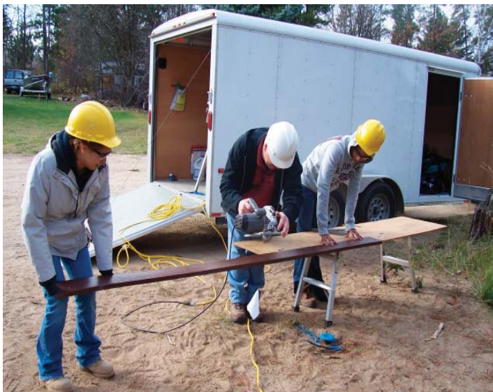
Photo above: Youthbuilders assist with cutting the siding for a new house.
