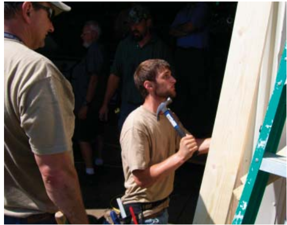
Cody constructs a new garage door at Central Minnesota Habitat for Humanity’s new location.
