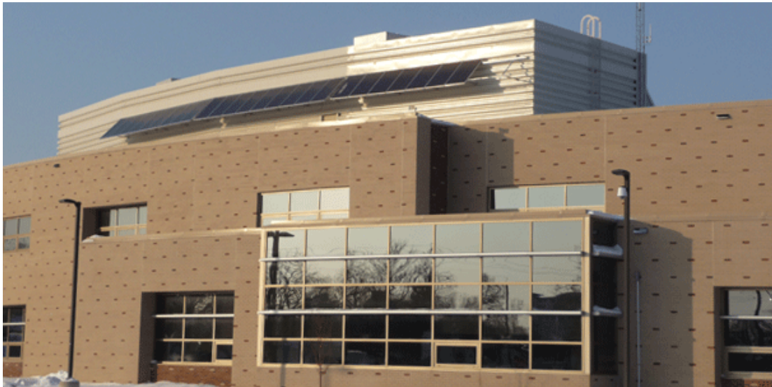
Mayo High School 5.8 kW PV system. Photo credit: Minnesota Student Energy Project
