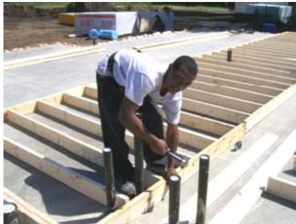
Youthbuilder Jameo, lays out an external wall at a Central Minnesota Habitat for Humanity twin home in the city of St. Cloud
