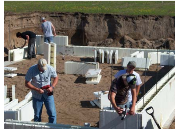
Perham Youthbuilders working on the foundation of the new housing construction site in the Perham Westwind Addition
