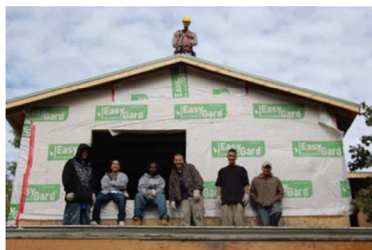
GAP Youthbuilders renovating a 19 th century farm house for affordable homeownership on St. Paul's west-side
