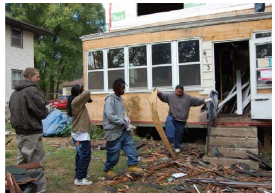
GAP Youthbuilders renovating 19th century farmhouse for affordable housing in St. Paul
