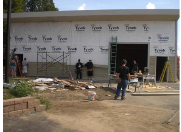
Youthbuilders installing siding on a large storage building newly constructed for Chanhassen High School
