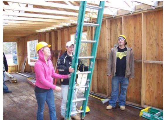
Youthbuilders, Lois Usher, John Jay, and Tyler secure a ladder during new construction of home in the city of Bemidji to be sold as affordable housing
