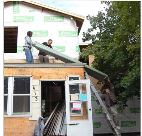
Youthbuilders hauling metal sheaths to be installed on the rooftop of 415 Robie Street in St. Paul
