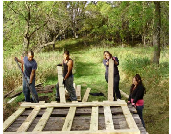
Miguel, Luis, Zaida and Valerie assist in the reconstruction of a dock for the Prairie Woods Environmental Learning Center in Spicer.
