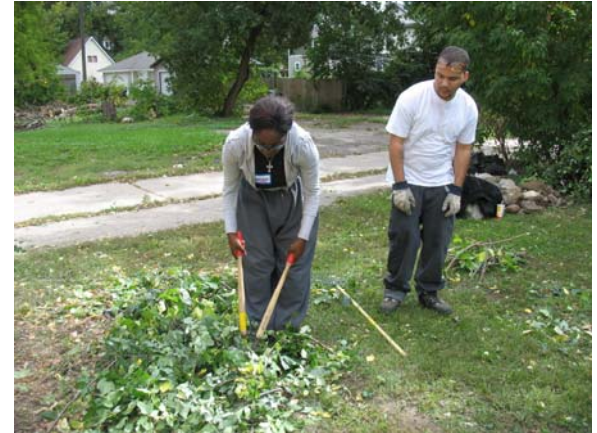
Nakinski and Dwight remove trees and brush at a home in north Minneapolis to prepare the property for construction
