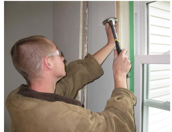
Albert installed trim boards along with new energy efficient windows in a renovated home in Chisholm
