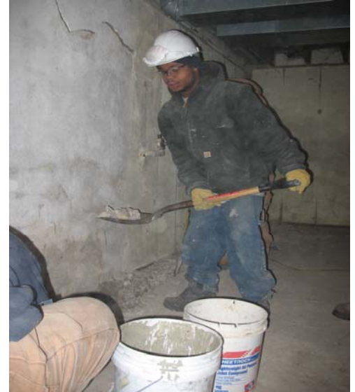
Tree Trust Youthbuilder, Kareem, removes broken concrete in the basement of a home under renovation through Urban Homeworks in North Minneapolis
