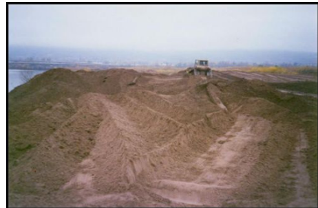
A bulldozer at Erie Pier moves dredged material to ready it for reuse. The material was hydraulically sorted
