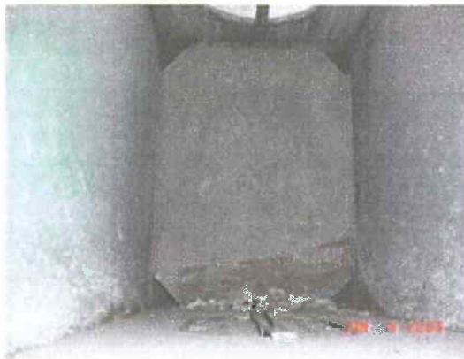
Back Side of Internal Diaphragm (Appears Welded)
